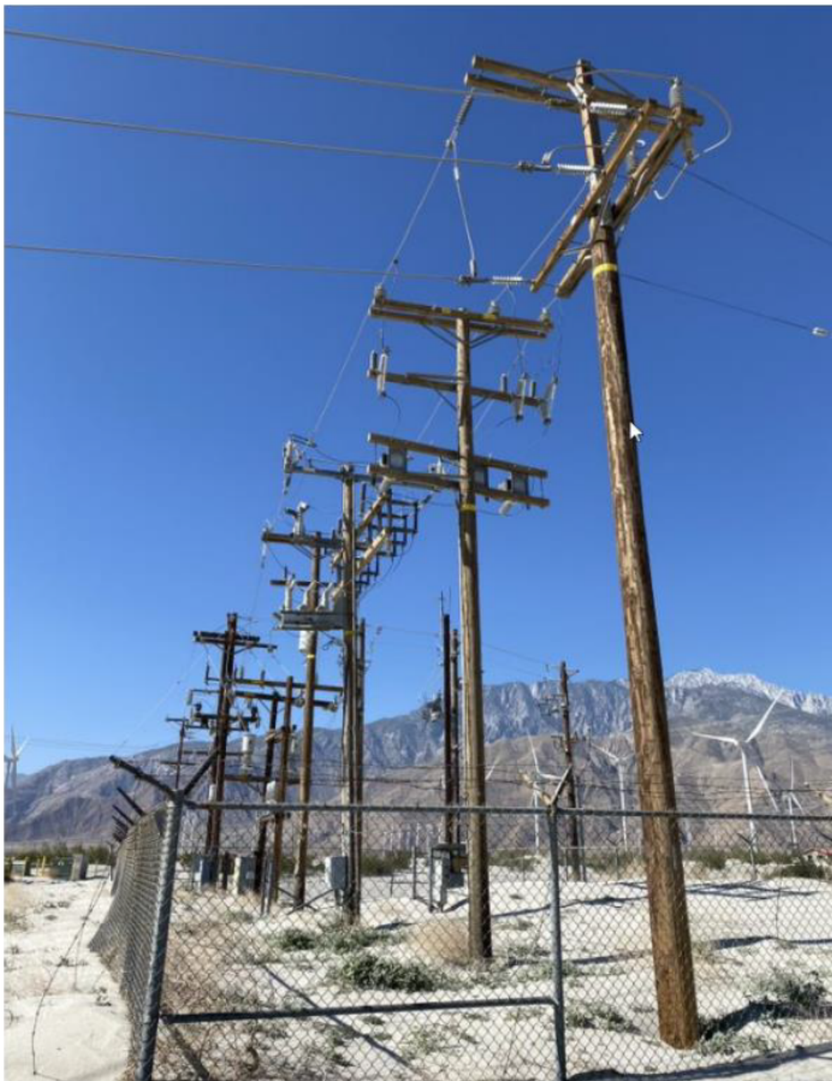
Figure 6: Photo of chain link fence to be removed and the general location of trenching. Photo is facing southwest
