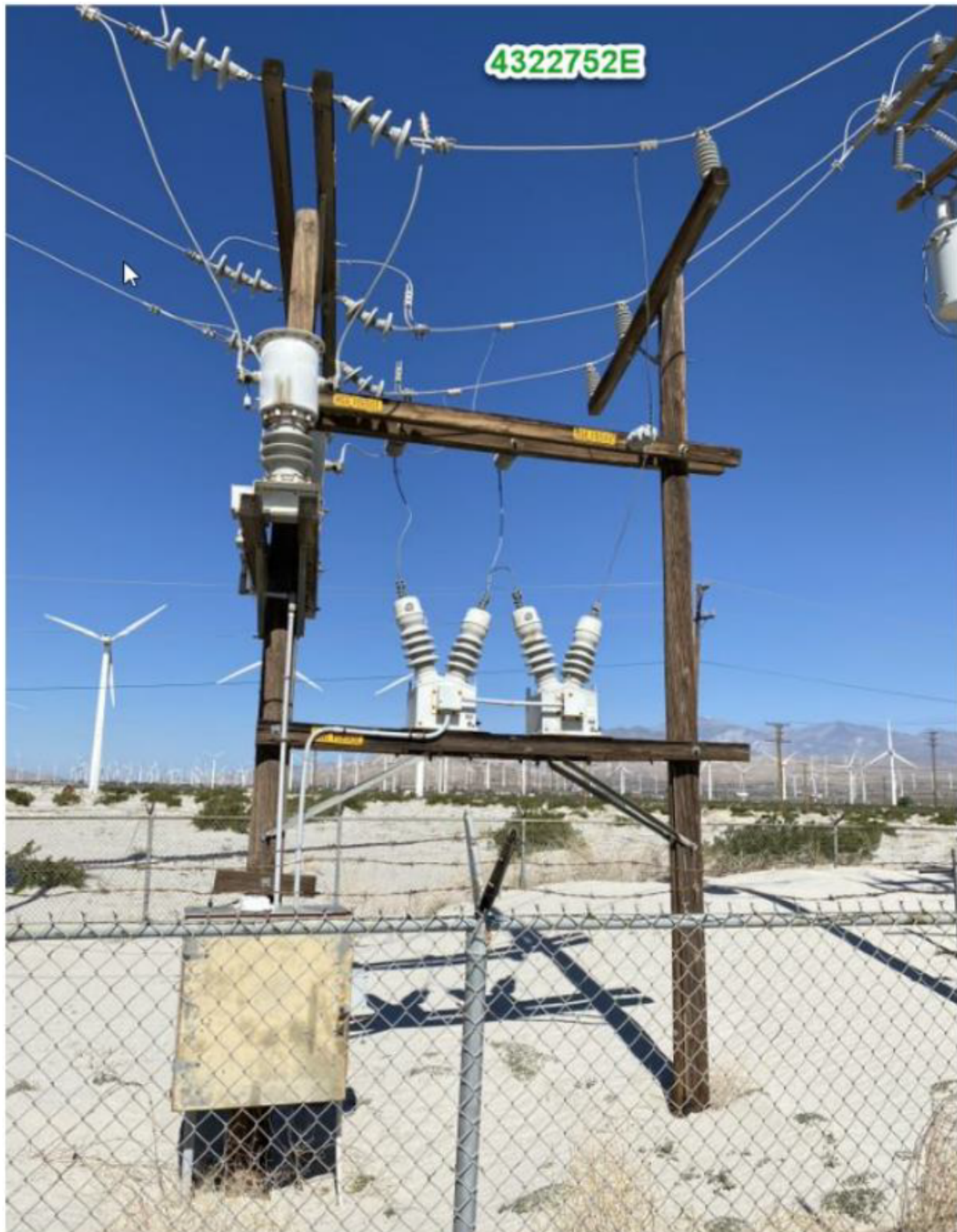
Figure 5: Photo of Pole 4322752E (wooden two-pole structure) and chain link fence to be removed. Photo is facing west.
