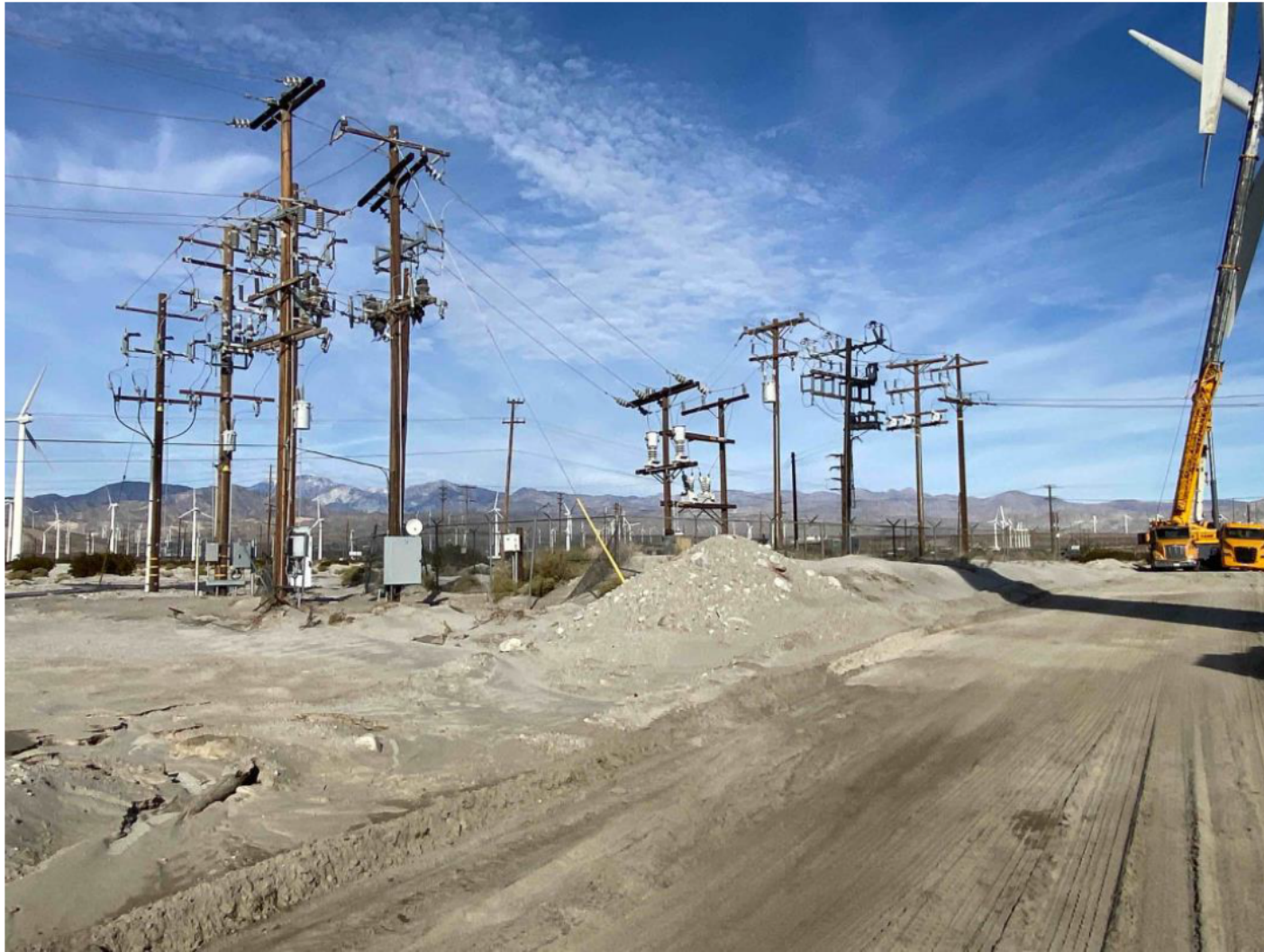
Figure 7: Photo of Project area showing Pole 4322752E and existing access road. Photo is facing northwest.
