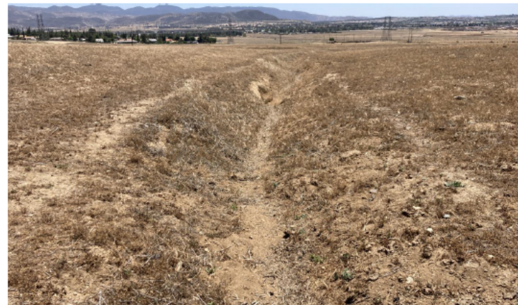
Photograph 8: View of Drainage I looking south.
