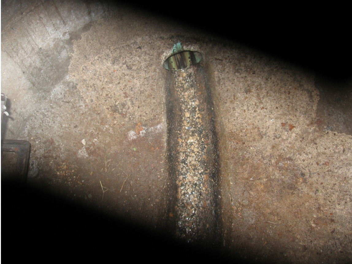
Sewer corrosion below a coffee shop
