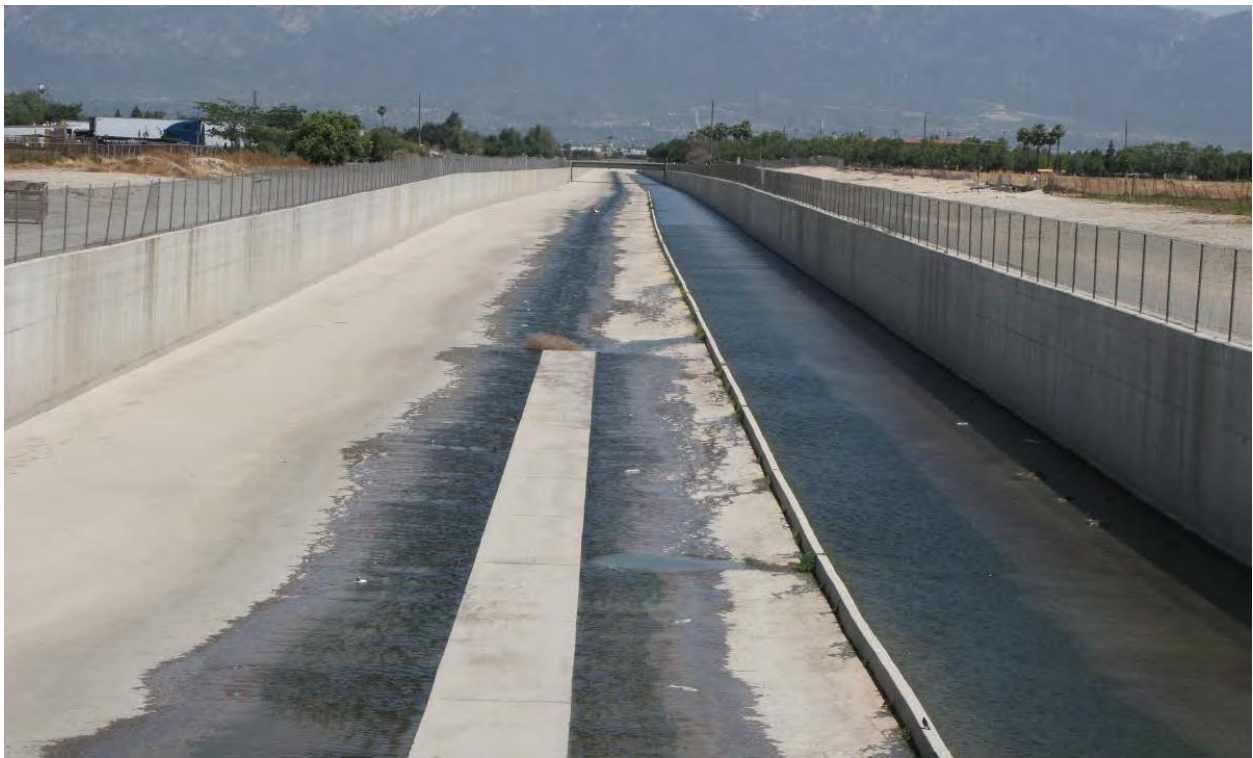
Figure CC-6. Reach 1 looking upstream. Eleven miles of the total 15 mile length of Reach 1 is contained by concrete vertical walls at 12-15 ft in height. (UAA Analysis CC)
