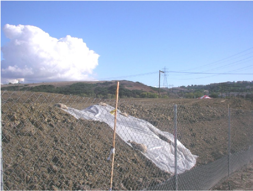
Photo 5 Plastic Spillway For Sediment Trap (Facing Southeast)
