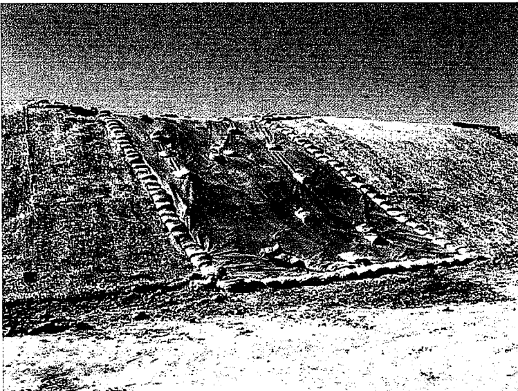
Photo 14. Stabilized spillway needs additional BMPs at the bottom of the slope and to get the water to the channel without causing erosion.
