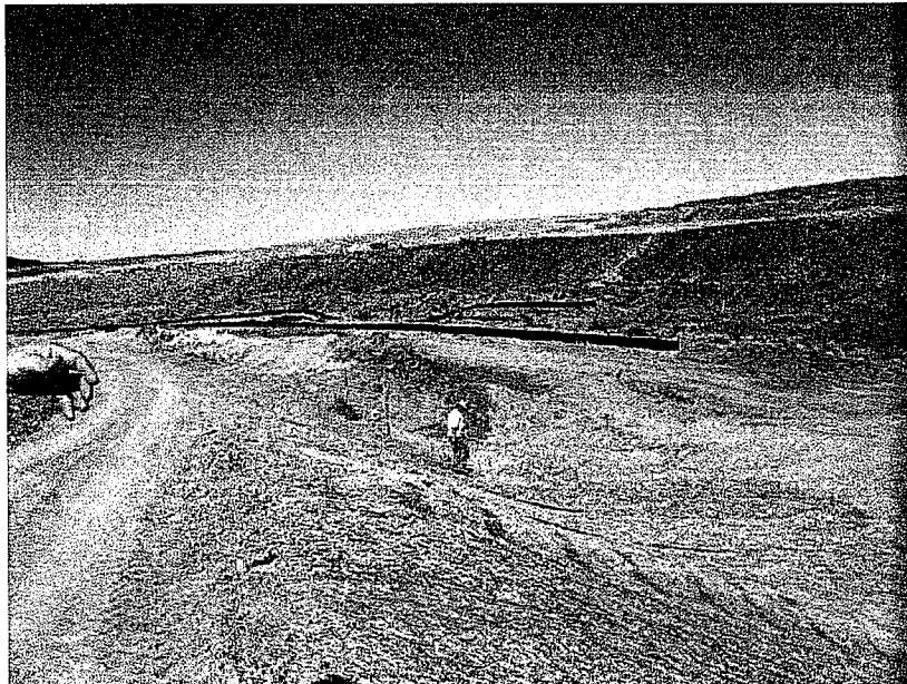
Photo 13. Access road into channel needs stabilization before a storm.
