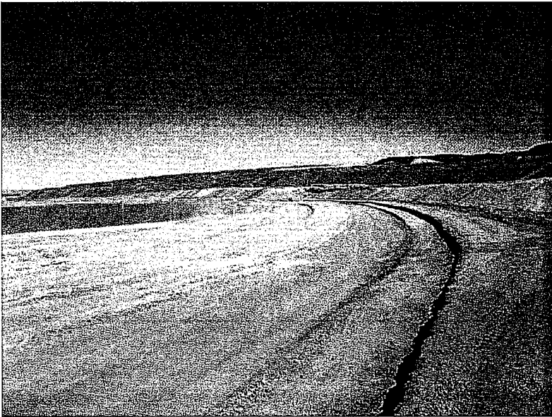
Photo 5. Top of completed bridge at Loop Road over Long Valley Wash. Bridge is a low point for water to accumulate. Additional BMPs are needed to prevent concentrated flow along road from causing erosion.
