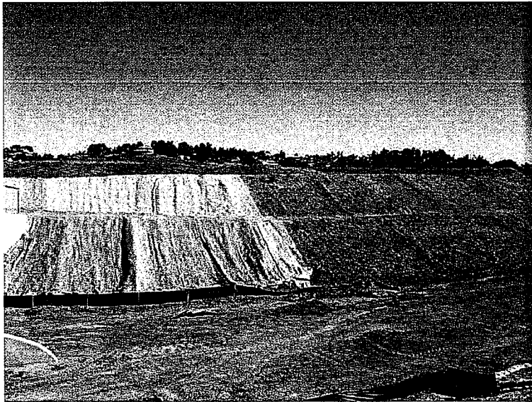
Photo 10. North bank upstream of Loop Road bridge. Some slopes have matting places and some slopes need to be stabilized.
