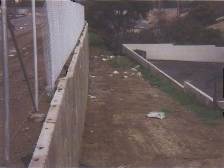
013. Excessive trash on the construction site.
