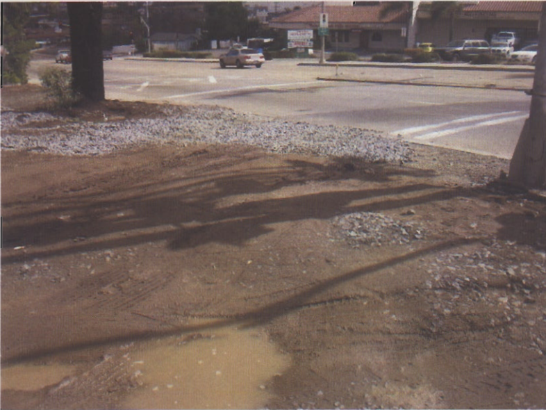
010. Inadequate gravel to prevent sediment tracking onto the adjacent Escondido Avenue.
