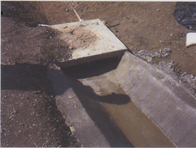
038. Sediment and sediment laden water discharge into a storm drain inlet without any inlet protection. This inlet is across the rail road tracks from the inlet in photo 037.
