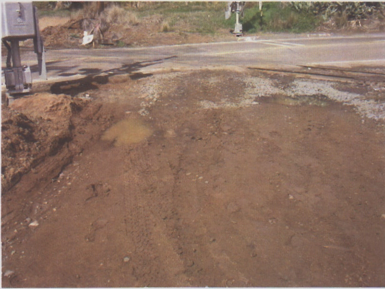
029. Inadequate gravel to prevent sediment tracking onto the adjacent street.
