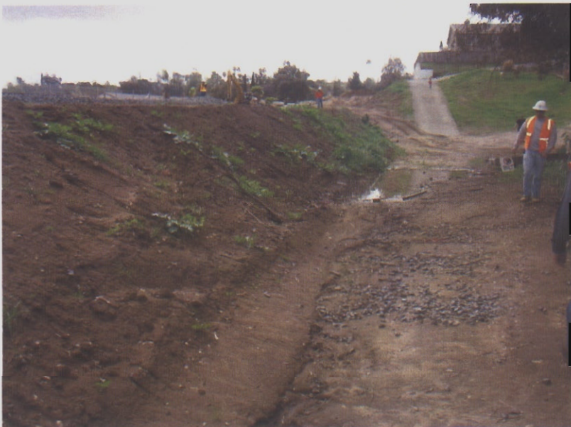
018. A long slope with no erosion or sediment controls.
