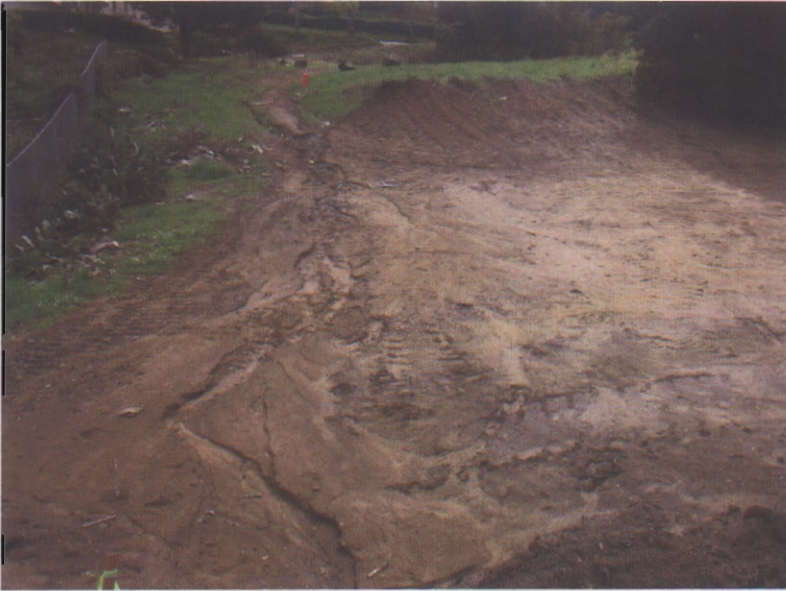
007. Erosion gully in a disturbed area without sediment or erosion controls.
