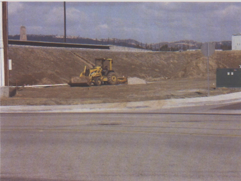
040. Sediment tracking onto the pavement. Slope behind the front loader is without erosion or sediment controls. No sediment controls behind the curb.
