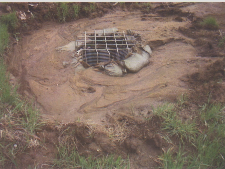
022. Sediment discharge at a storm drain inlet that is completely overwhelmed from sediment flows. This inlet received runoff from the material storage yard that has soil stabilization and sediment controls.
