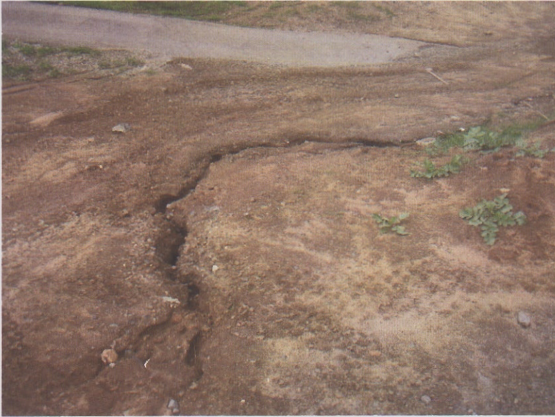
015. Another erosion gully in an area without erosion controls.
