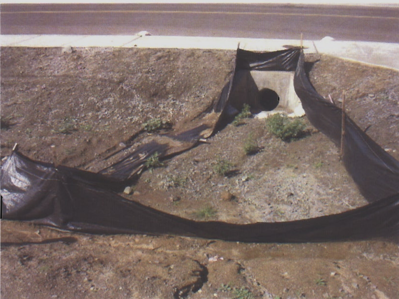
034. Sediment discharge at a storm drain inlet without adequate protections. Silt fence has been overwhelmed due to a lack of upstream source control measures.
