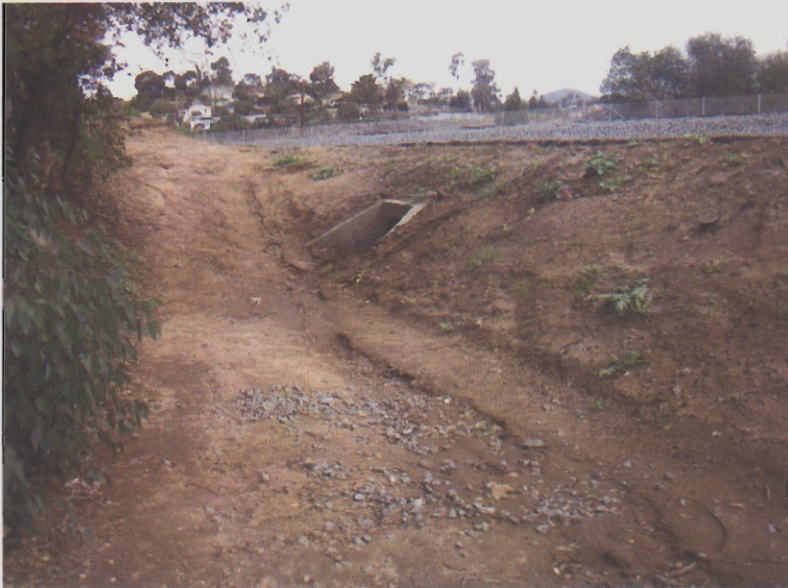
016. Storm drain discharge point with no energy dissipation.
