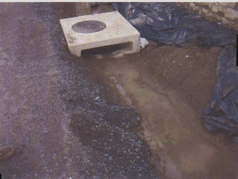
037. Sediment and sediment laden water discharge at an unprotected storm drain inlet.
