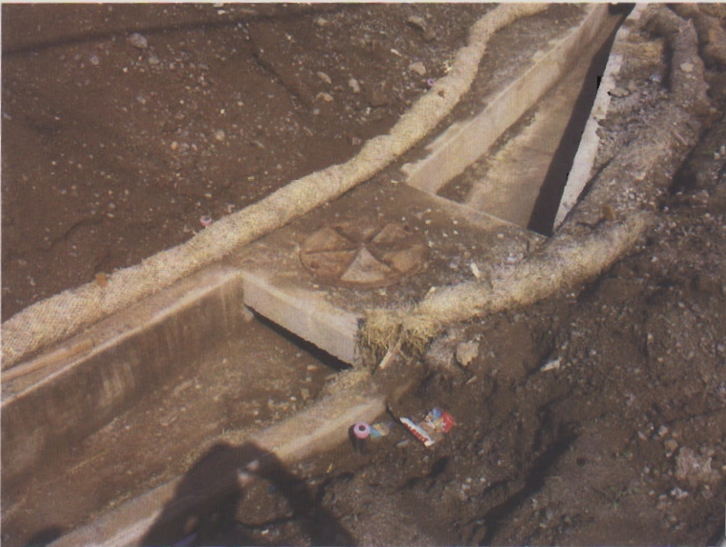
033. Sediment discharge into a storm drain inlet without any inlet protections. Fiber rolls are deteriorated and not placed properly. Slope is without erosion controls.
