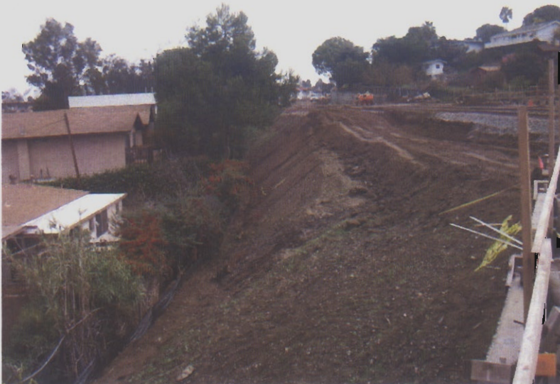
006. A large slope without erosion control measures.
