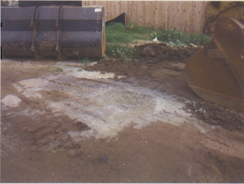
012. Another concrete slurry spill not far from the one in photo 011.
