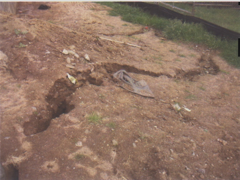
014. Erosion gully down a slope with no erosion controls.
