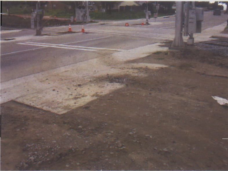
019. Sediment tracking onto the adjacent paved surface due to a total lack of BMPs.
