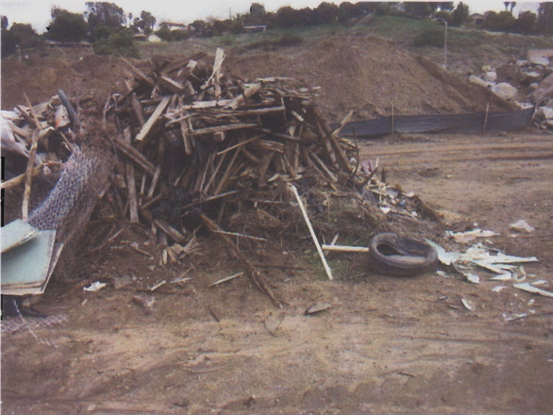
024. Construction trash storage is inadequate with no containment or coverage.
