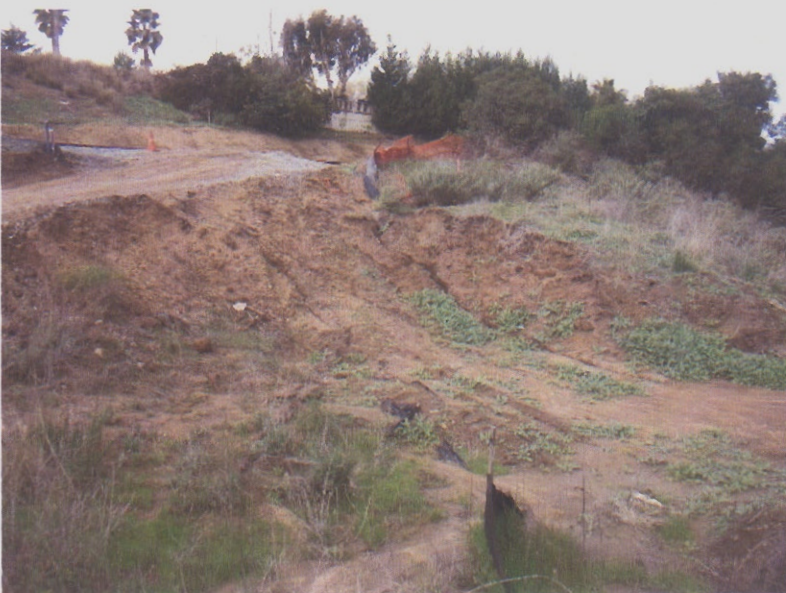
025. A slope is without adequate erosion or sediment controls is eroding away. Silt fencing is inadequate, not maintained and overwhelmed.
