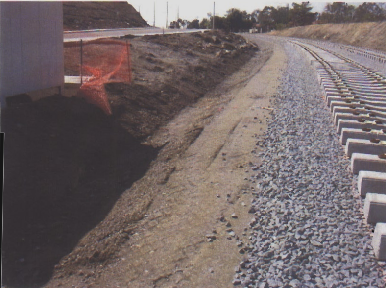
036. Upstream of photo 035 there is a lack of sediment or erosion control BMPs.
