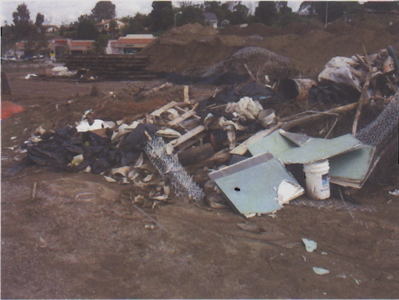
023. Construction trash storage is inadequate with no containment or coverage.
