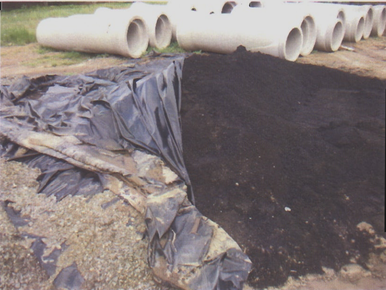
021. Although this asphalt stockpile does have plastic to cover it in case of rain, site personnel did not cover the stockpile. Puddles of water are seen on top of the folded up plastic.
