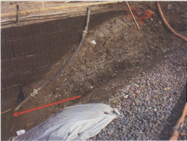
026. Bare dirt next to the bridge abutments is eroding away and discharging into Buena Creek. The arrow points to the edge of the creek.
