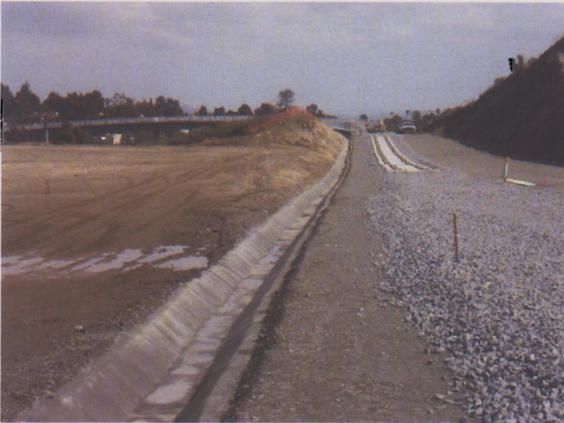
039. Storm drain channel without any perimeter sediment controls.
