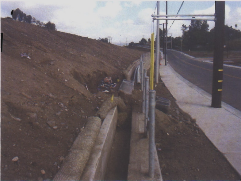
032. A large slope is without any erosion control protections. Dirt is stockpiled in the storm drain ditch.
