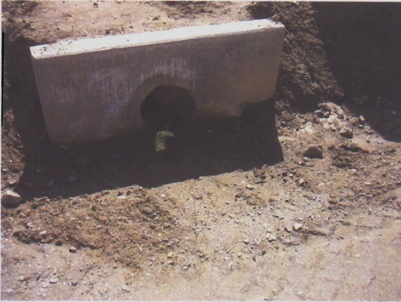
035. Sediment discharge at a storm drain inlet without any inlet protections.
