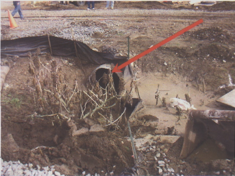
005. Storm drain inlet is without adequate protections. Silt fence is completely overwhelmed and failing resulting in a discharge of sediment into the storm drain inlet.
