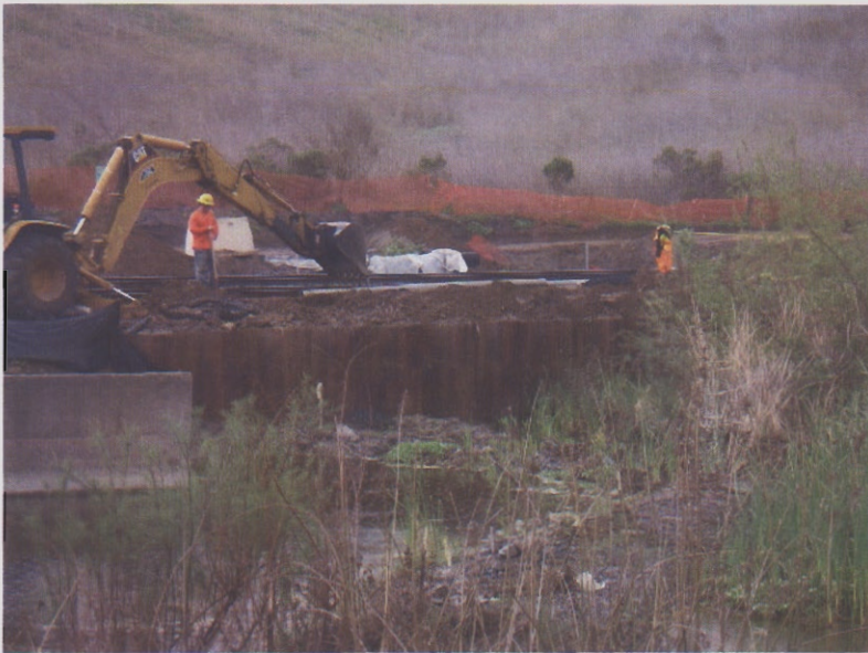
7. Construction work next to Loma Alta Creek causes sediment to spill into the creek. No sediment controls are at the top of the wall.
