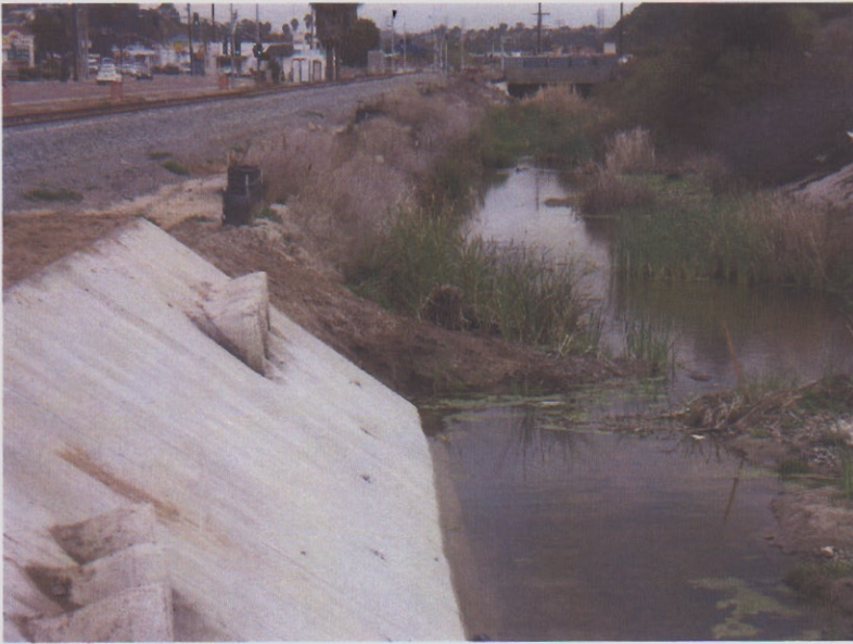
4. Sediment discharge to Loma Alta Creek.
