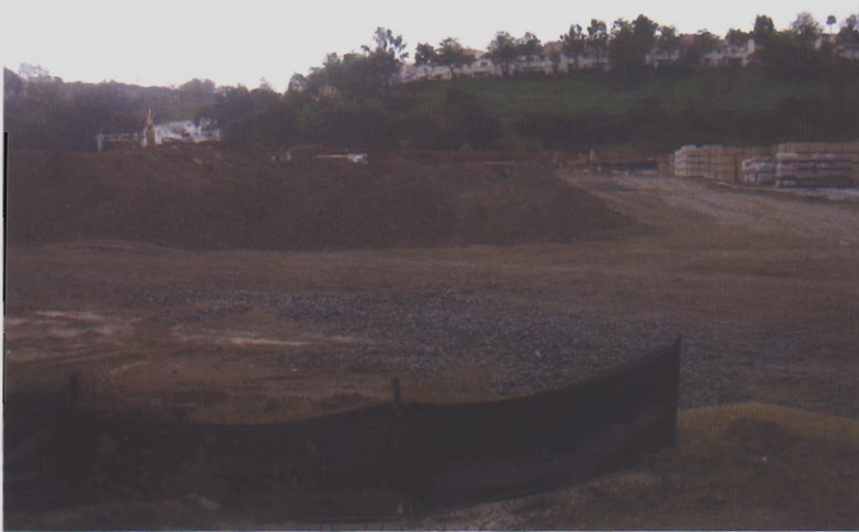
10. Soil stockpiles with no cover or containment.
