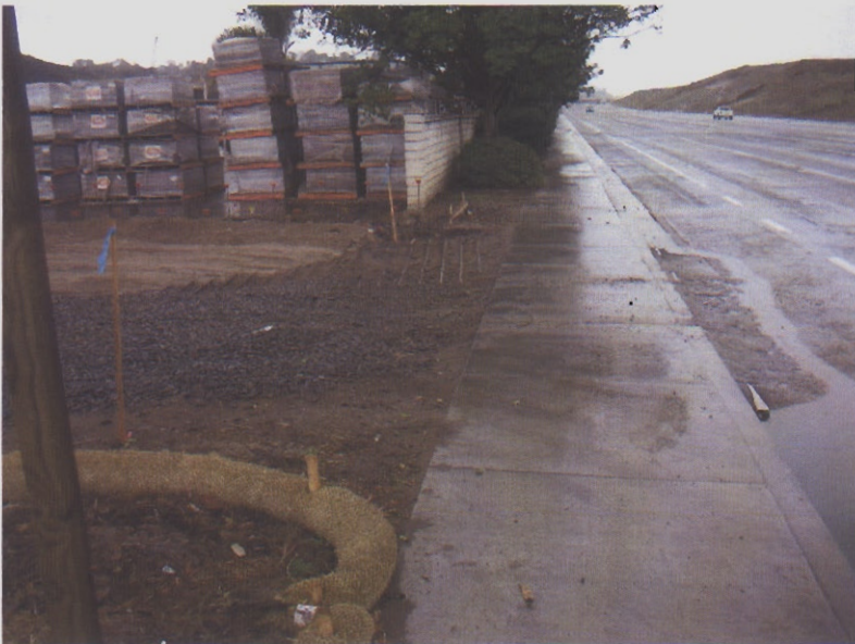
11. Construction exit with inadequate gravel to prevent sediment tracking.
