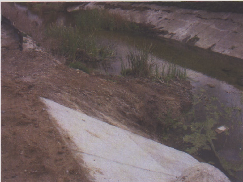
5. A closer look at the sediment discharge. Silt fence at the top of the bank stops right at the sediment discharge.
