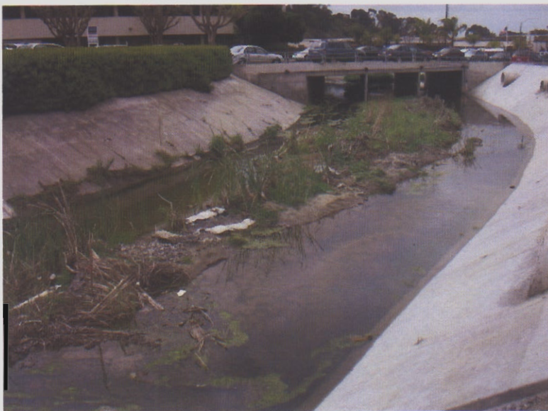
6. Looking downstream from the sediment discharge, gravel bags are in the creek.
