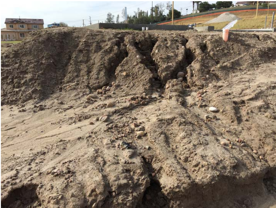
Figure 5. Failure to implement erosion control BMPs on inactive areas.
