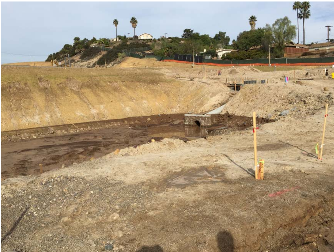
Figure 8. Failure to apply linear sediment controls. Photograph taken by Wayne Chiu, San Diego Water Board, on December 15, 2014, depicting the lack of linear sediment controls on a slope. IMG_5035.jpg
