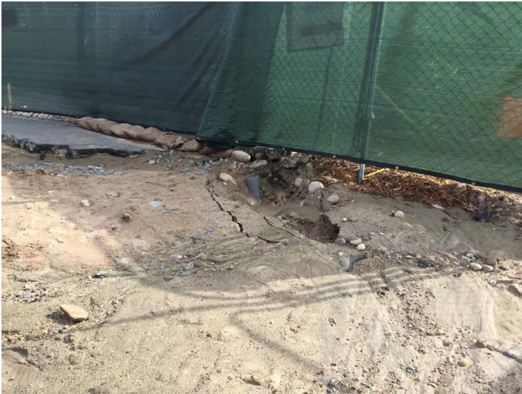
Figure 9. Failure to manage run-on and runoff. Photograph taken by Wayne Chiu, San Diego Water Board on December 15, 2014, displaying erosion caused by runoff flowing under fence and offsite. IMG_5042.jpg.
