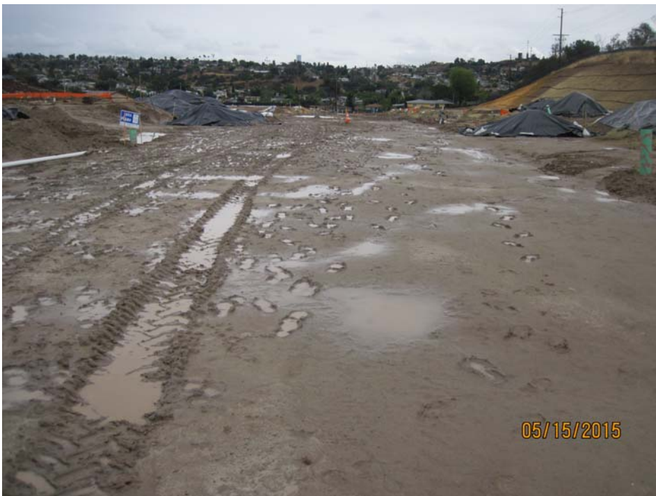
Figure 7. Lack of erosion control BMPs in active areas. Photograph on May 15, 2015, of muddy thoroughfare (Tangelos Place) lacking erosion control BMPs after rain event. Photograph taken by Frank Melbourn, San Diego Water Board. IMG_0354.jpg
