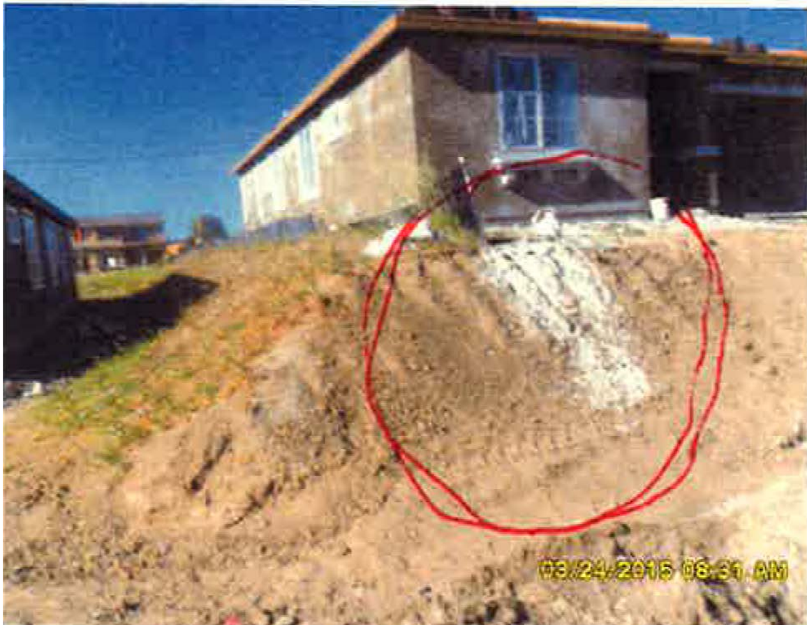
Figure 13. Failure to prevent the discharge of concrete waste to the ground. Photograph taken by the City of Lemon Grove on March 24, 2015, depicting discharge of concrete waste on slope (identified by red circle).
