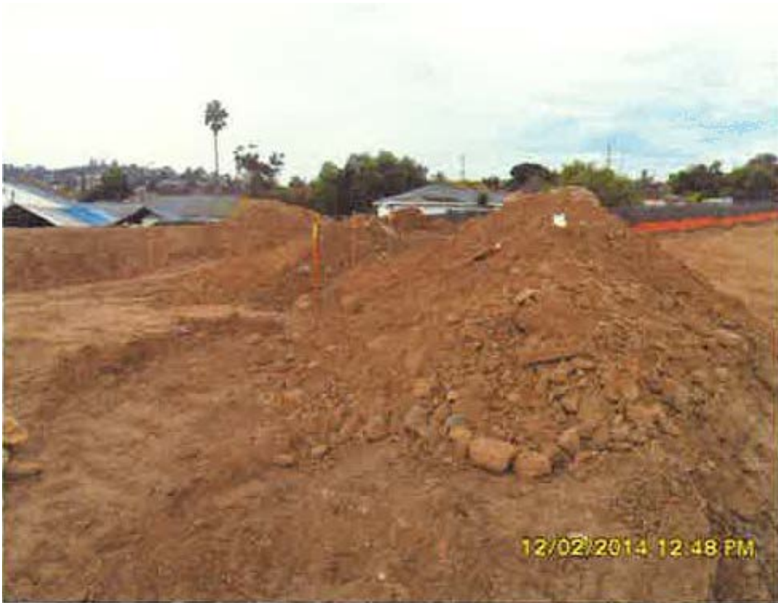
Figure 3. Failure to implement material stockpile BMPs. Photograph taken by the City of Lemon Grove on December 2, 2014.
