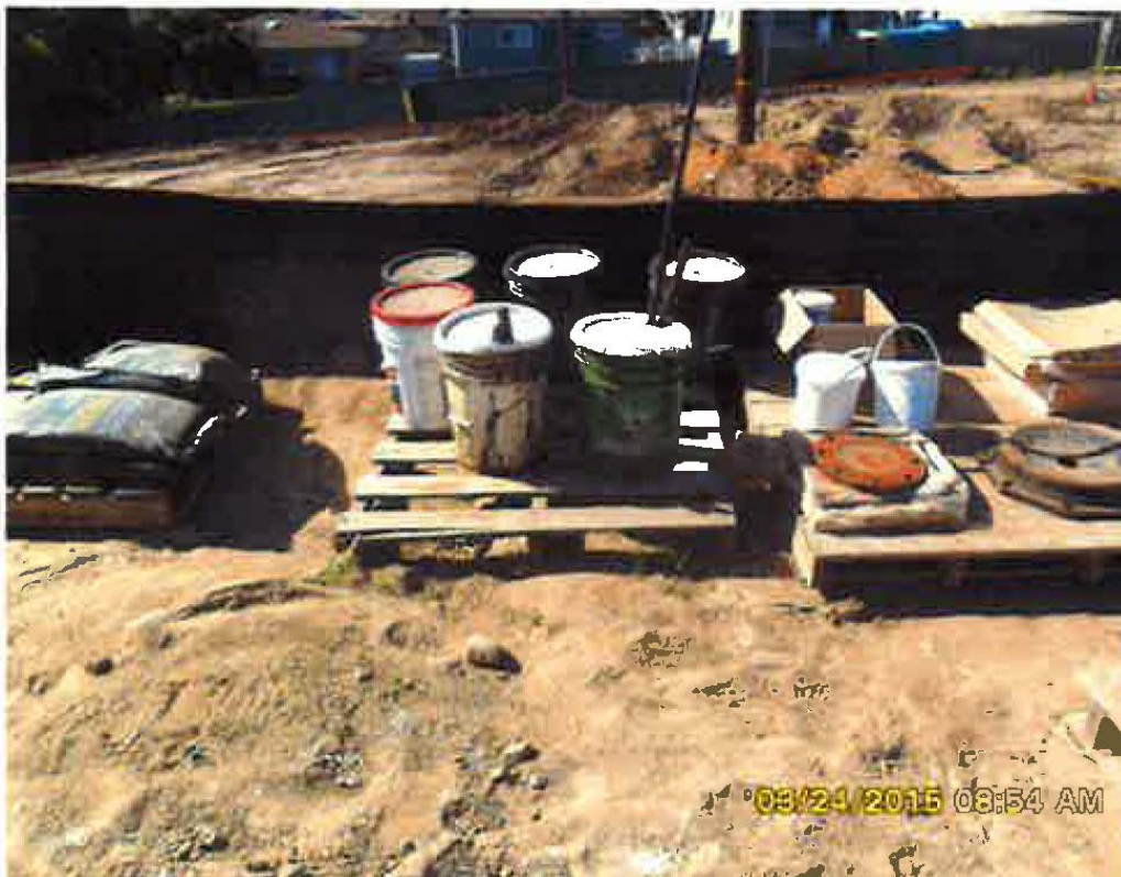
Figure 12. Failure to properly store chemicals. Photograph taken by the City of Lemon Grove on March 24, 2015, depicting chemicals and vehicle lubricants stored on pallets without protection from the elements and without secondary containment.
