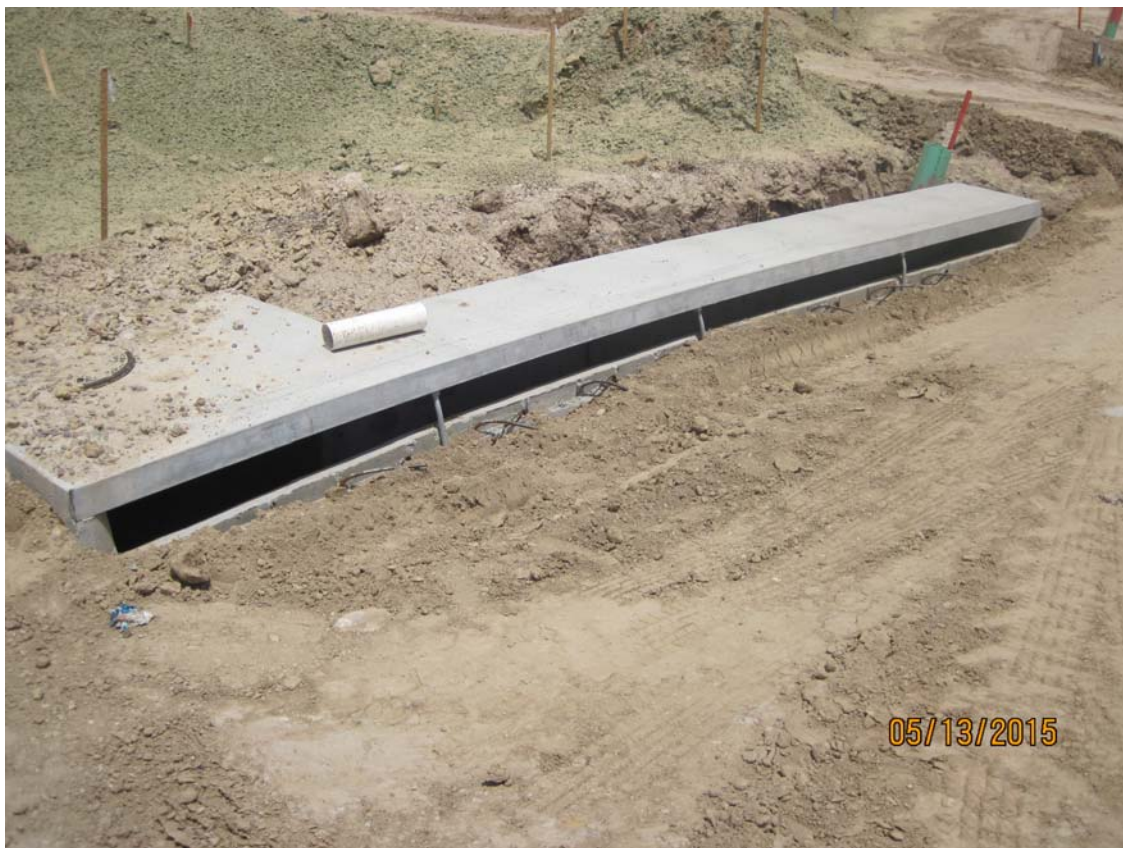
Figure 11. Failure to protect storm drain inlets. Photograph taken by Frank Melbourn, San Diego Water Board on May 13, 2015, displaying unprotected storm drain inlet. IMG_0295.jpg.
