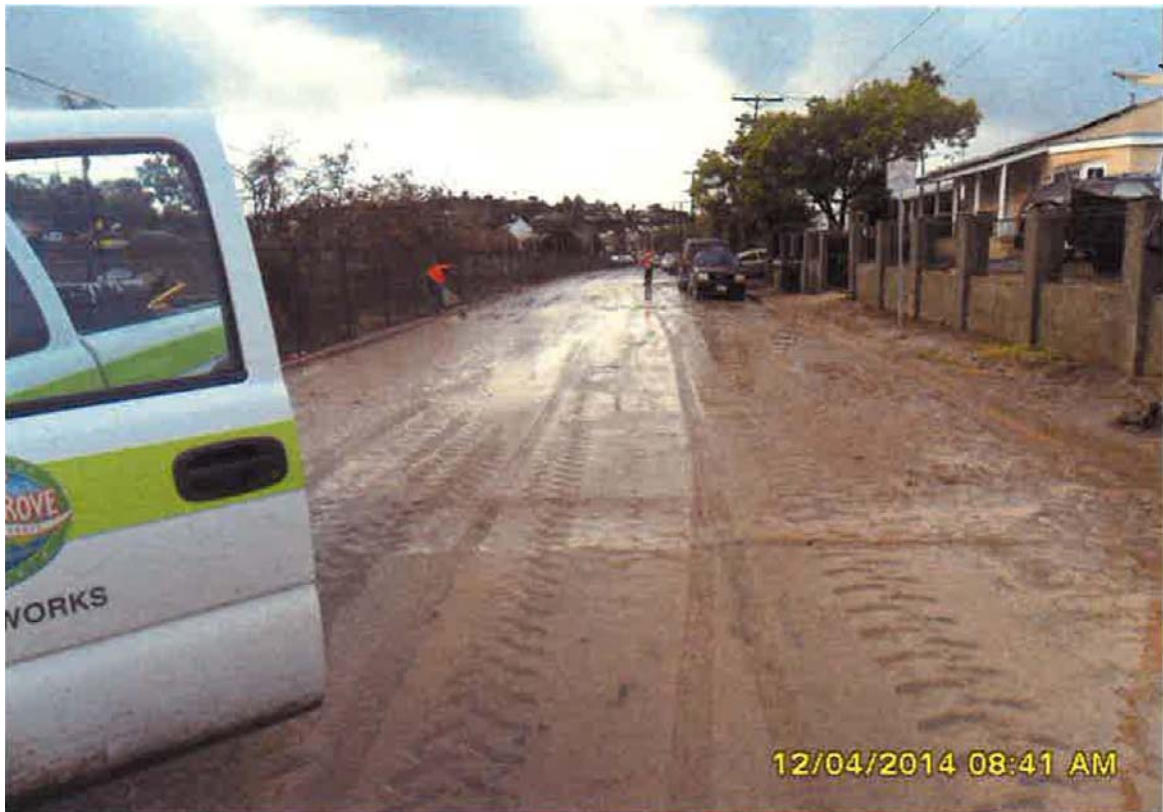
Figure 10. Failure to remove sediment from roads. Photograph taken by the City of Lemon Grove on December 4, 2014, depicting sediment on Akins Avenue southwest of the Site.
