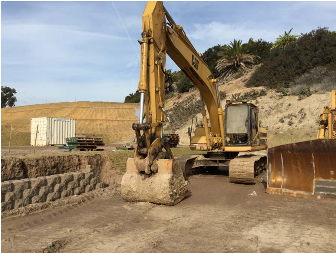
Figure 4. Failure to have vehicle fluid leak protection. Photograph taken by Wayne Chiu, San Diego Water Board on December 15, 2014, of heavy equipment without vehicle fluid leak protection. IMG_5064.jpg
