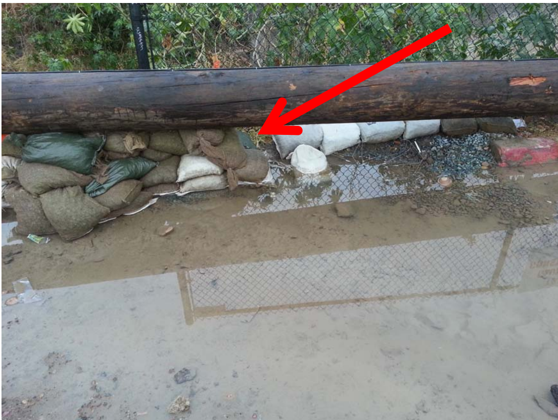
Figure 6. Failure to implement perimeter sediment control BMPs. Photograph taken by Frank Melbourn, San Diego Water Board on May 8, 2015, of gap (identified by red arrow) in perimeter sediment control BMPs that resulted in sediment discharge to Encanto Channel. 20150508_192234.jpg
