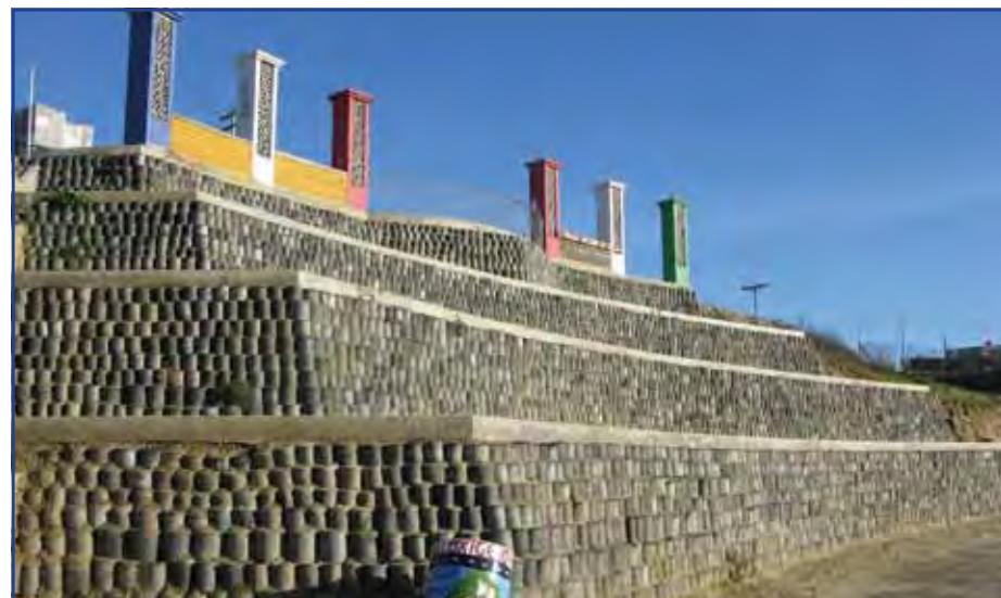
Construction of retaining walls using waste tires may be a way to beneficially reuse waste and reduce sources of trash
