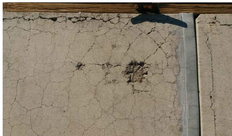
TYPICAL SURFACE SPALL ⑤ SCALE: NTS
