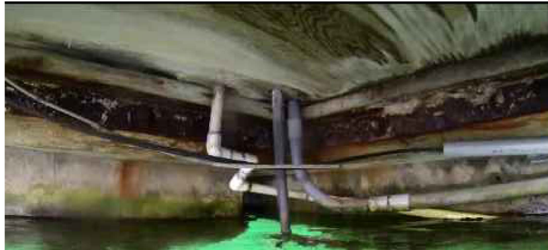
CORRODED AND DELAMINATED ANGLE FRAME ②
