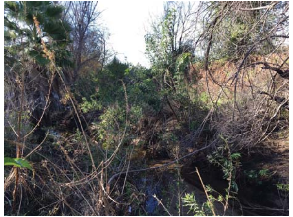
Figure 7. Additional view looking downstream. Deeply incised northwest bank is visible.
