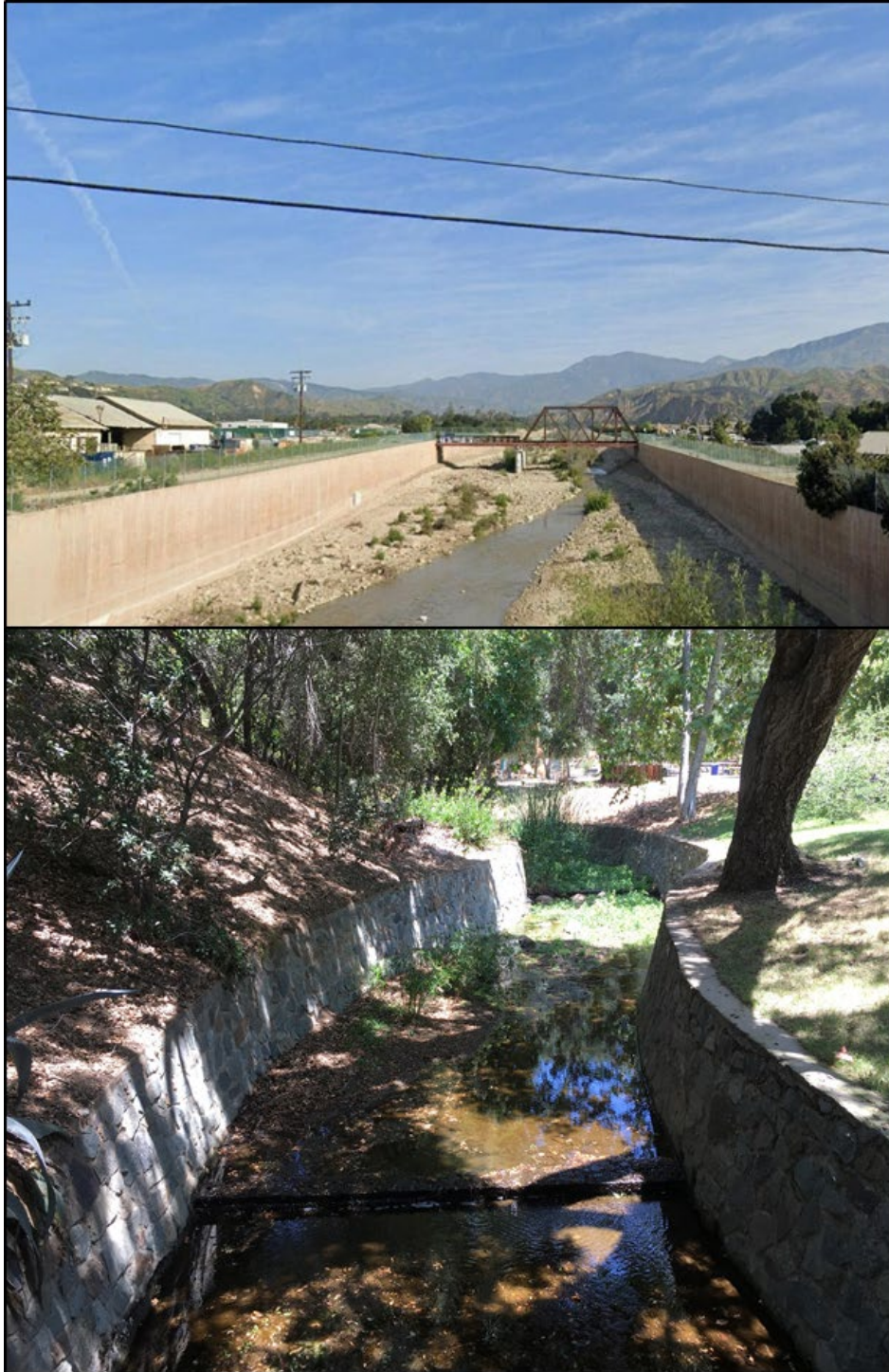
Figure 15. Examples of stream segments that have modified features but are not physically hardened from bank to bank (i.e., hardened streambed segments). These streams have physically hardened stream banks but retain a natural stream bottom. These stream segments have CSCI scores that would meet the Stream Biological Objective. Top: Santa Paula Creek (CSCI: 0.94, 0.99). Bottom: Los Cocheros Creek (CSCI: 0.85).
