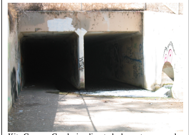
Kit Carson Creek is diverted downstream under North County Fair. Flow here is about 3 cfs.
