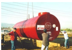
Underground storage tank
