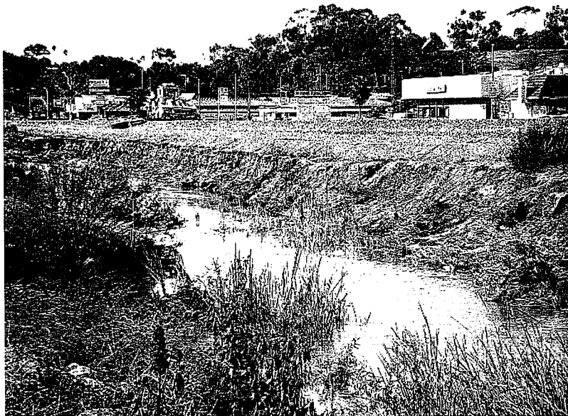
26. Loma Alta Creek has eroded away on the north bank threatening the tracks. A sediment discharge occurred. Workers were moving the tracks away from the eroded embankment. Photo looks Northwest.
