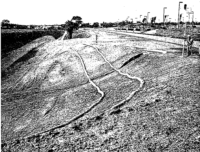
20. A side view of the gully erosion in photo 17. The erosion was caused by concentrated storm water runoff flowing down the slope. Photo looking West.
