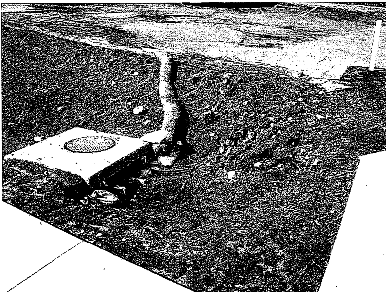
33. Another view of the inlet in photo 31 shows the opposite side of the inlet. The slope has erosion gullies. Sediment has overtopped the gravel bags resulting in a sediment discharge. Photo looks North west.
