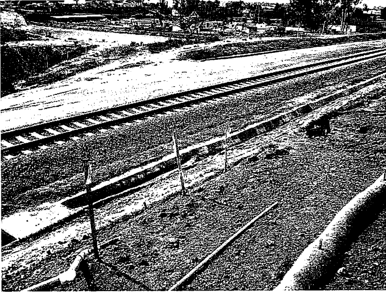
16. Mud from the erosion in photo 15 has entered the storm drain channel. Photo looking south west.
