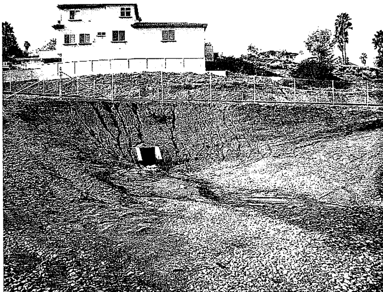
11. Another slope with erosion gullies has no erosion controls. Concentrated storm water runoff from the culvert flows through the construction yard. Photo looks South.
