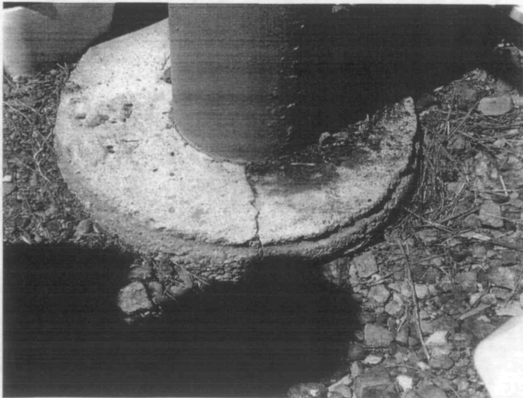
Photo 8 – SMGW-35, Crack in Well Seal.
