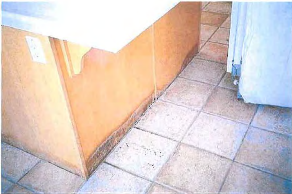
Photo 4- water migration through slab into cabinetry
