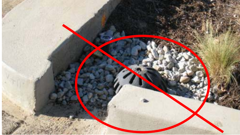
Figure 6: Incorrect Placement of an Overflow Inlet.
