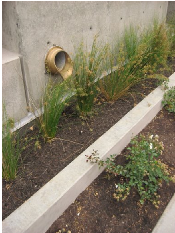
Figure 9. Disconnected downspout discharging to planter box.
