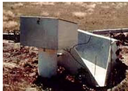
H-flume (with Instrument Shelter)
