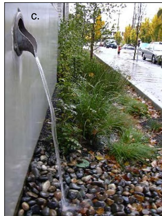
Figure 3: Runoff from larger rooftops can be treated in cisterns (a), infiltration areas (b), or bioretention planting beds (c).
