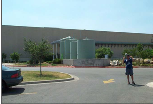
Figure 1b: Large Building Cistern System, Austin, TX
