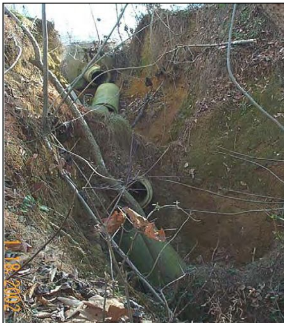
Figure 5: Reconstruction and/or bioengineering may be needed to stabilize outfalls that discharge down steep slopes.
