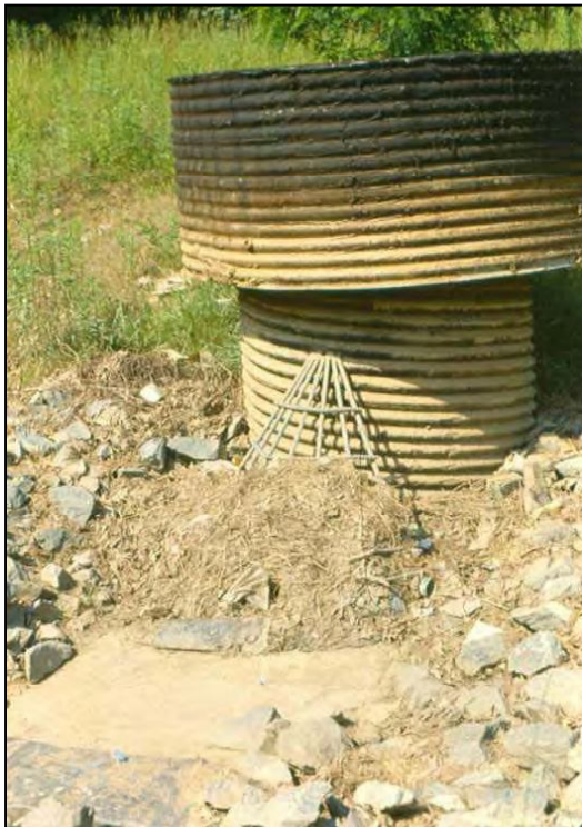
Figure 8: Designers should anticipate clogging problems by woody debris at crossing retrofits.
