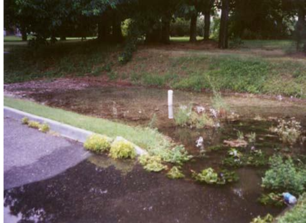
Figure 1: Failed Infiltration Trench
