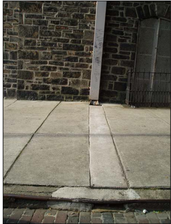
Figure 1: Downspout from St. Martin Church on Fayette.
