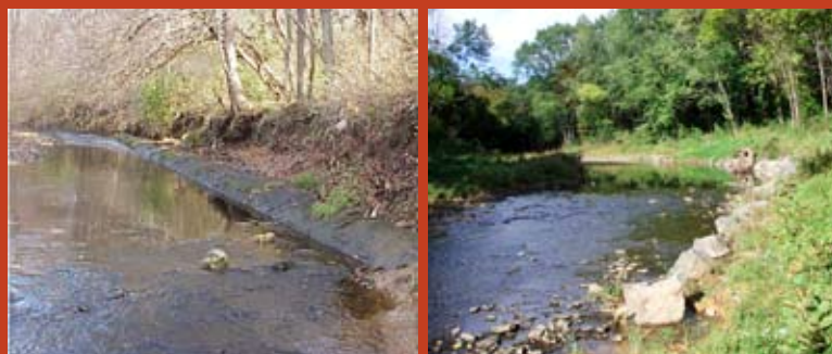
Before and after a stream restoration of exposed interceptor pipe along Marshall Road in the Cobbs Creek Watershed.
