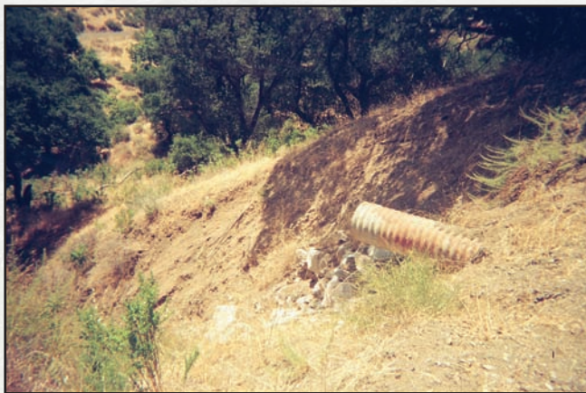
Figure 5.2—Shotgun culverts causes accelerated erosion.
