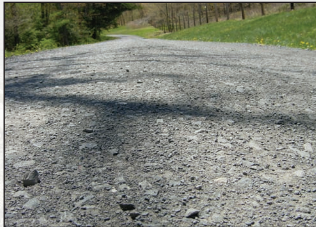
Figure 8.3—3-year-old dense packed surface aggregate after 40,000 vehicles.
