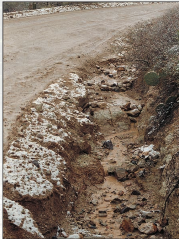
Figure 4.6—Eroded ditches are a common problem.
