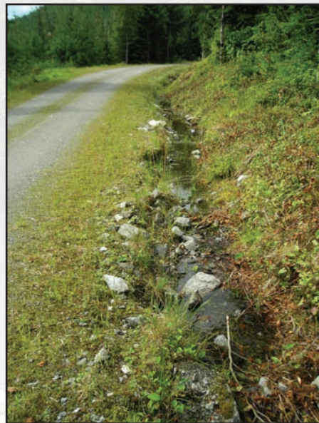
Figure 2.4—Road ditch with standing water.
