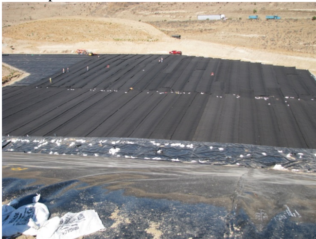
Figure 1: The new Stage III-C unit at Sycamore Landfill. The view is from the top of the sideslope looking down to the base of the unit.
