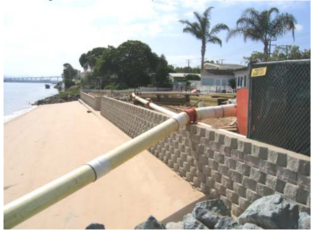
Figure 2. Post construction shoreline condition, with un-permitted seawall construction, and discharge of fill material (beach sand)
