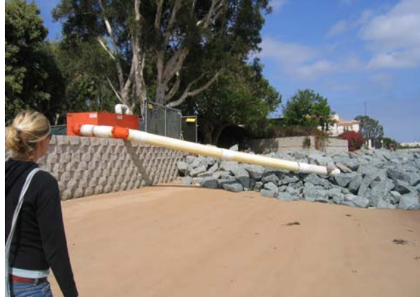
Figure 6. It is unknown what the pipe shown here is discharging offsite into City of Coronado Project footprint (possibly used to spread sand on constructed beach?)
