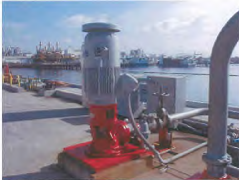
Figure 1. Main Fire Pump on Pier Six.
