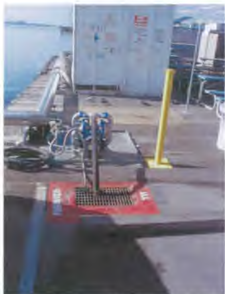
Figure 5. Storm Water Collection System Pump.
