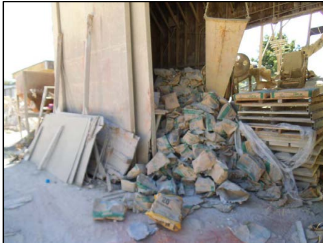
San Diego Water Board staff observed multiple instances where poor storage of materials could lead to the runoff of pollutants. Photo by San Diego Water Board.
