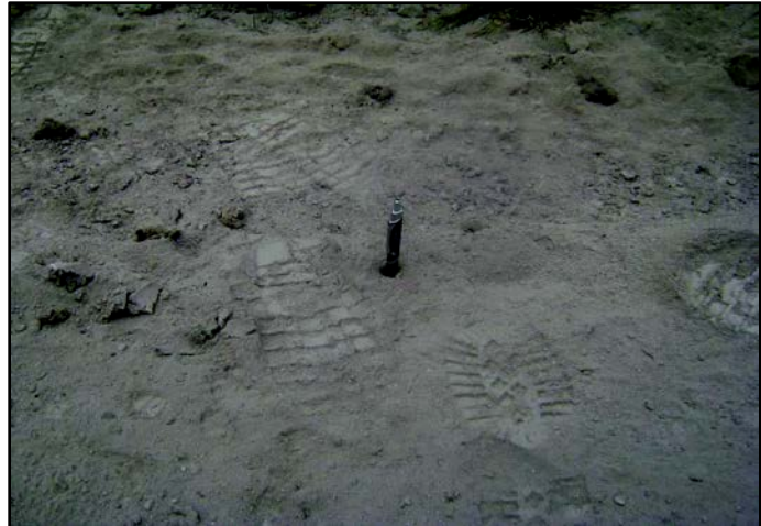
San Diego Water Board staff observed 2 to 3 inches of concrete/cement powder on the ground. It was so thick staff could place a pen in the dust and have it stand up on its own. Photo by San Diego Water Board
