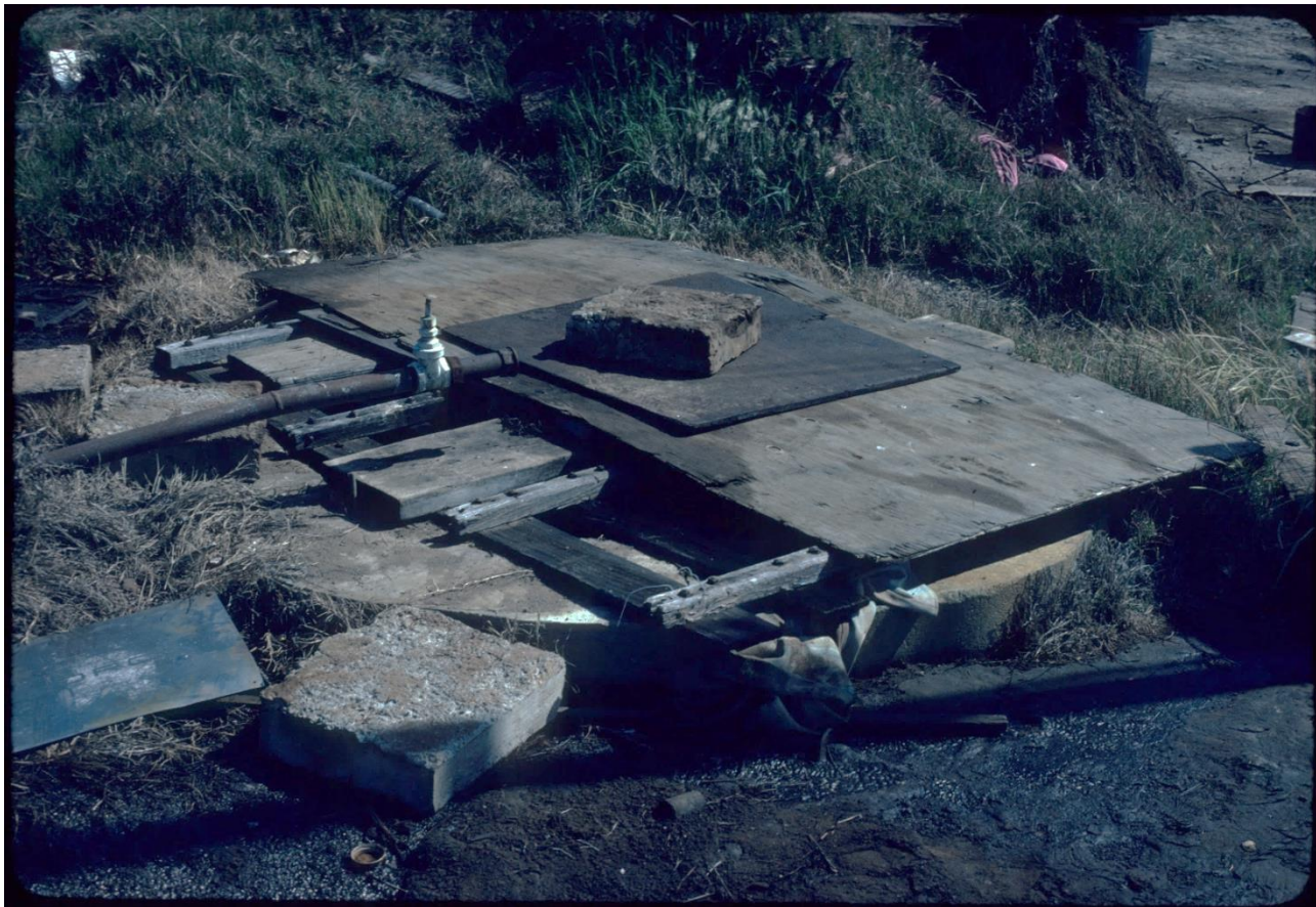
Figure 2. Photo taken in April 1982 of the well head cover over the 65-foot well showing chemical staining on the cover and on the ground.
