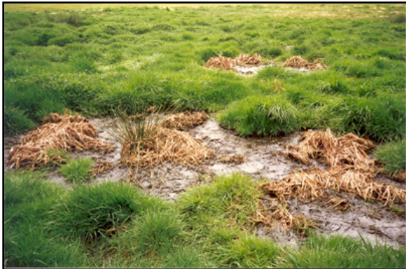
Effluent rising to the surface above a septic tank or leach field is one sign of septic system failure.
