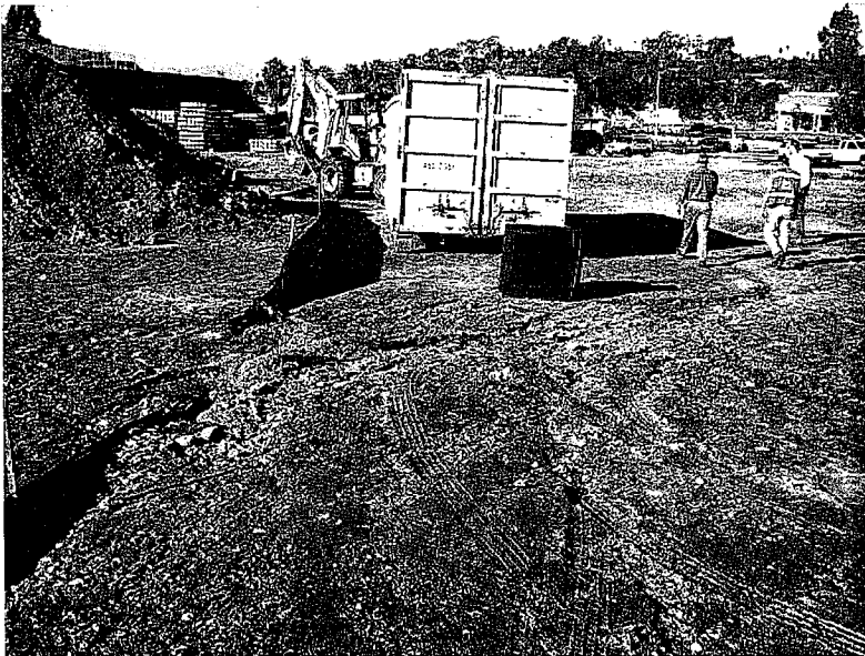
8. Silt fence has failed around this soil stockpile.
