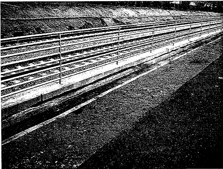
14. Slopes on left side of picture exhibit hydroseeded areas that have slumped or sloughed off of the slope. Bare soil on the right side of picture lacks adequate stabilization.
