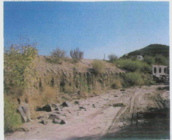
Figure 6. Rip-rap fill and erosion of the Northern bank downstream of culvert.
