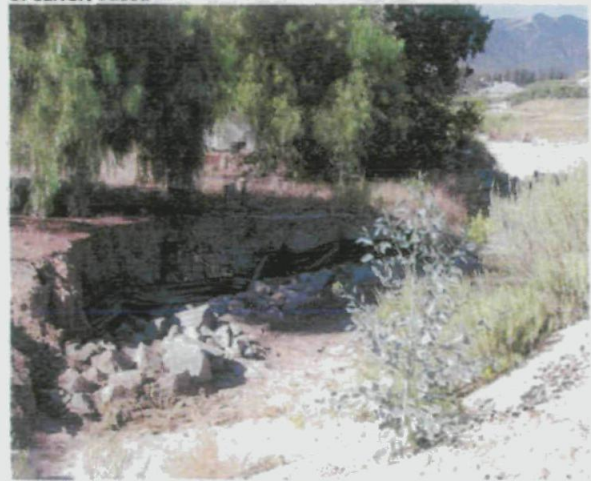
Figure 4. Rip-rap fill and erosion of Southern bank downstream of culvert outlet.
