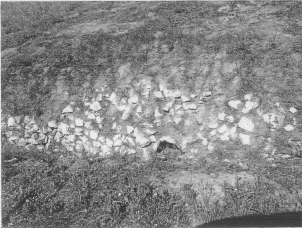
Sediment in drainage culvert.
