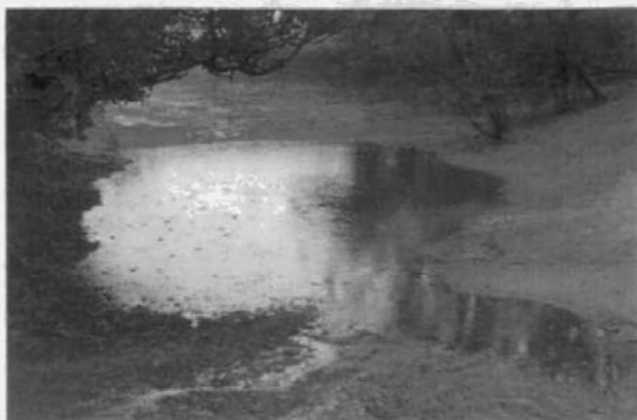
Photograph 1 – ASL cover ponding
