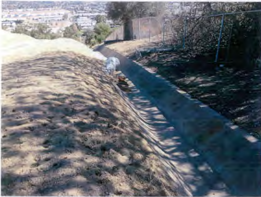
Figure 3- Southern Perimeter Drainage Channel
