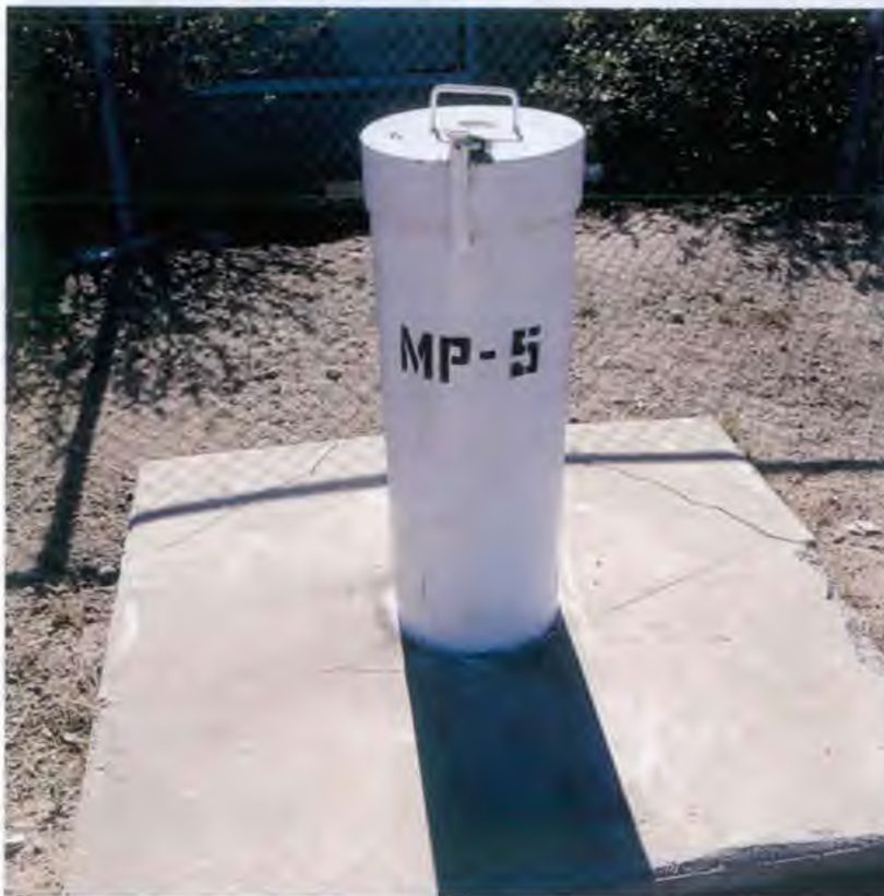
Figure 4- Landfill Gas Monitoring Probe MP-5
