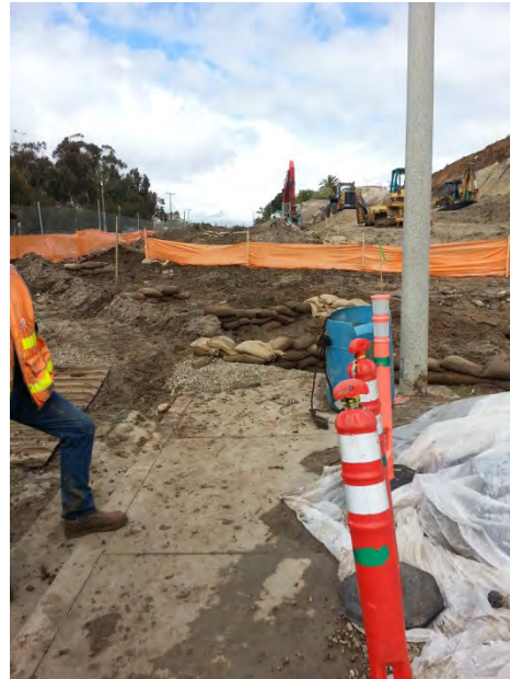
Photo 6: Check dams installed after rain event. Evidence of sediment discharged on the sidewalk. Discharge the result of lack of, insufficient amount, and ineffective installation of check dams and no silt fence prior to rain event. See Attachment No. 1 - 3-02-15 City of Carlsbad Incident Summary Photo at 0745 and 0930.
