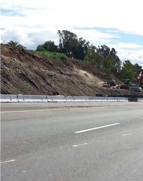
Photo 3: Project site located east of El Camino Real. Slopes unprotected from erosion. Soil stabilizer(s) not in place. Linear sediment controls not in place. (view is east along El Camino Real at the north end of the site at 1130 hours).
