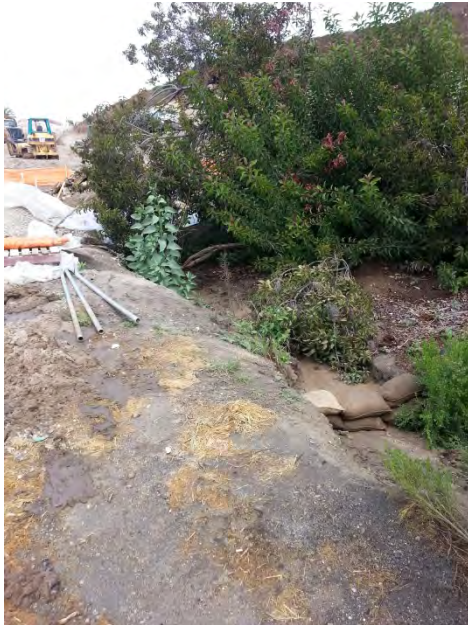
Photo 9 Lack of perimeter controls, inadequate run-on controls, lack of erosion in conjunction with sedimentation controls, and lack of soil stabilization controls resulted in a discharge of sediment and sediment laden water from the site. Discharge of sediment beyond the gravel bag dike and sediment deposited as seen in Photo 10 is evidence that sediment was discharged from the site to the unnamed tributary to Agua Hedionda Creek and Agua Hedionda Lagoon. (view is at south end of the site at the discharge point looking north).
