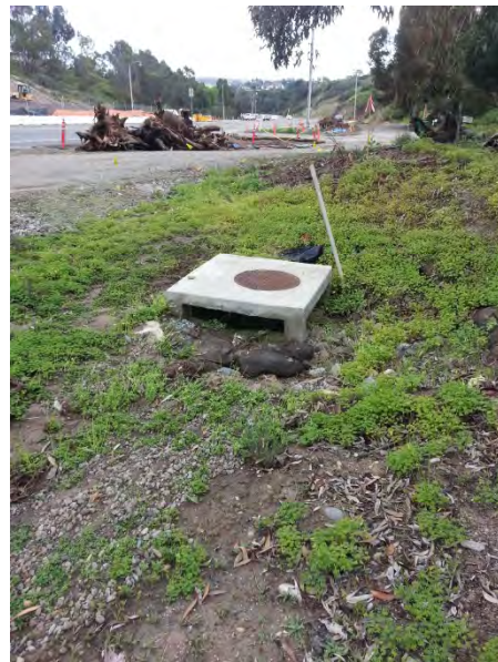
Photo 14 Unprotected inlet. This inlet is located directly down gradient of site shown in Photo 15. Erosion and sedimentation shown in Photos 13-15 are evidence of a discharge of sediment and sediment laden storm water to the MS4.
