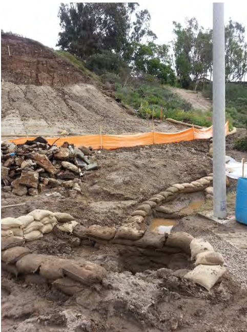
Photo 7 Sedimentation basin constructed after rain event. See Attachment No. 1 - 3-02-15 City of Carlsbad Incident Summary Photo at 0745 and 0930 – sedimentation basin not installed) Sedimentation basin not designed in accordance with CASQA Construction BMP Guidance Handbook as required by CGP.
