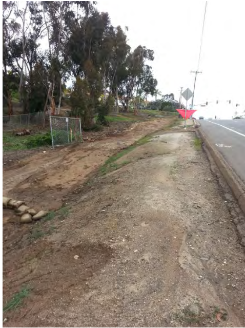
Photo 13 Lack of perimeter controls, lack of run-on controls, lack of erosion controls, lack of erosion controls in conjunction with sedimentation controls, and lack of soil stabilization controls. (view at north end of the site located on the west side of El Camino Real looking north).
