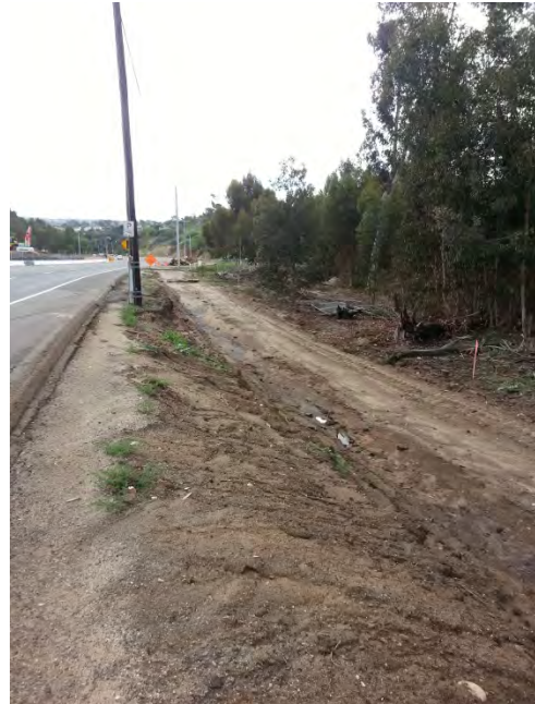
Photo 14 Lack of perimeter controls, lack of run-on controls, lack of erosion controls, lack of erosion controls in conjunction with sedimentation controls, and lack of soil stabilization controls. (view at north end of the site located on the west side of El Camino Real looking south).
