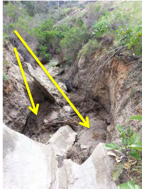
Photo 10 Discharge of sediment traveled along concrete v-ditch shown in Photo 9 to discharge to earthen bottom unnamed tributary as seen here to Agua Hedionda Creek and Agua Hedionda Lagoon. Photo Evidence shows discharge from the site caused or contributed to hydromodification in this receiving water. This project is also required to comply with San Diego Water Board Water Quality Certification 08C-074. (view south of the site, in the unnamed tributary to Agua Hedionda Creek and Agua Hedionda Lagoon at the point where the concrete v-ditch discharges into the earth bottom receiving water).
