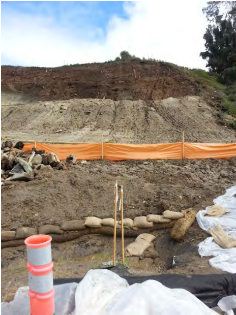
Photo 5: Project site slopes unprotected from erosion. Soil stabilizer(s) not in place. Linear sediment controls not in place. Silt fence and gravel bag berms installed after rain event (See Attachment No. 1 - 3-02-15 City of Carlsbad Incident Summary Photo at 0745 and 0930 – silt fence not installed) (view is east perpendicular to El Camino Real at the south end of the site at 1130 hours).
