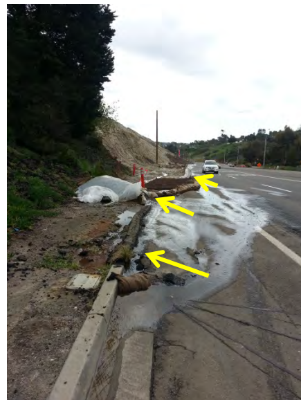
Photo 12 Ineffective perimeter controls and protection from run-on. Storm water run-on flow pattern seen here. Breached perimeter and run-on controls shown by yellow line. Perimeter controls and run-on protection was reinforced after the rain event (See Attachment No. 1 - 3-02-15 City of Carlsbad Incident Summary Photo at 0745 and 0930)
