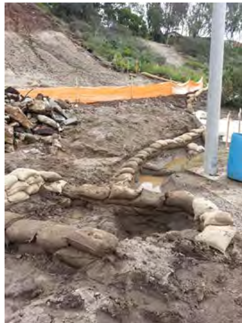
Photo 8: Sedimentation basin is extremely shallow and not designed in accordance with CASQA Construction BMP Guidance Handbook as required by CGP.
