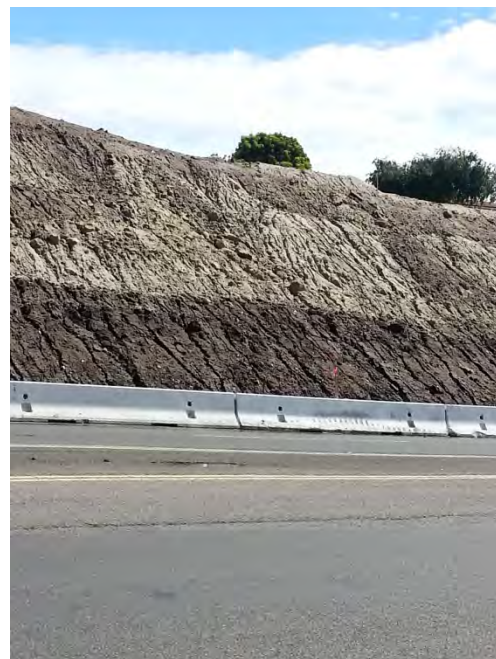
Photo 4: Evidence of significant erosion on steep slopes as the result of slopes being unprotected from erosion, of soil stabilizer(s) not being used, and failure to install linear sediment controls. (view is east along El Camino Real at the north end of the site at 1130 hours).
