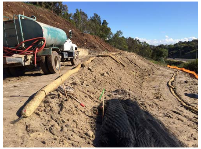
Time: 1500 By : D. Carlin View of project site near end of shift as crew began installation slope protection BMPs.
