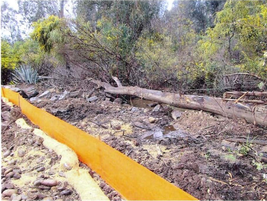
Photo 7 –Construction activities and debris have entered entering waters of the United States and/or State.
