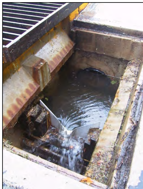
FIGURE 5-54 Weir flow used to measure flow rate. SOURCE: Robert Traver, Villanova University.
