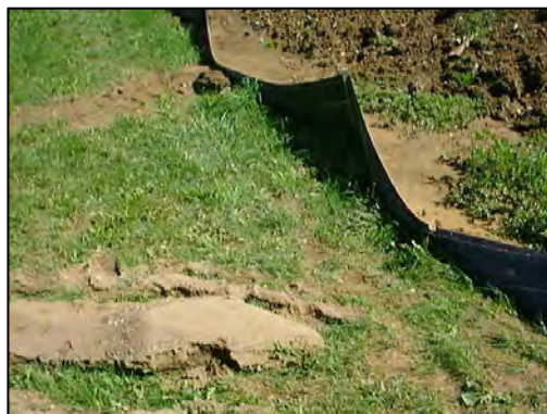
FIGURE 5-7 A functioning silt fence (top) and an improperly maintained silt fence (bottom). SOURCES: Top, EPA NPDES Menu of BMPs (available at http://cfpub.epa.gov/npdes/stormwater/menuofbmps/index.cfm?action=factsheet_results&view=specific&bmp=56 ) and, bottom, Robert Traver, Villanova University.
