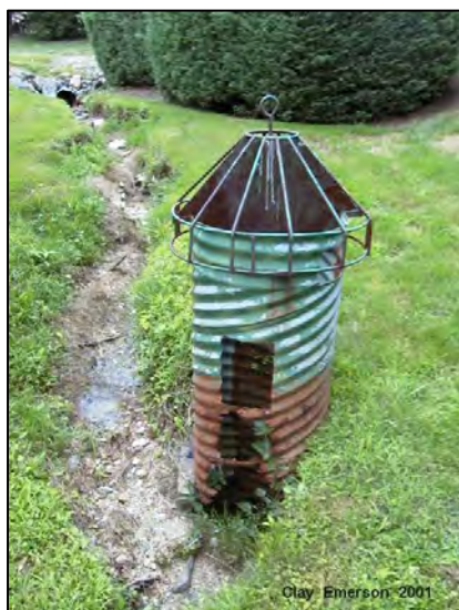
FIGURE 5-50 Rusted outlet structure. SOURCE: Reprinted, with permission, from Emerson. Copyright by Clay Emerson.
