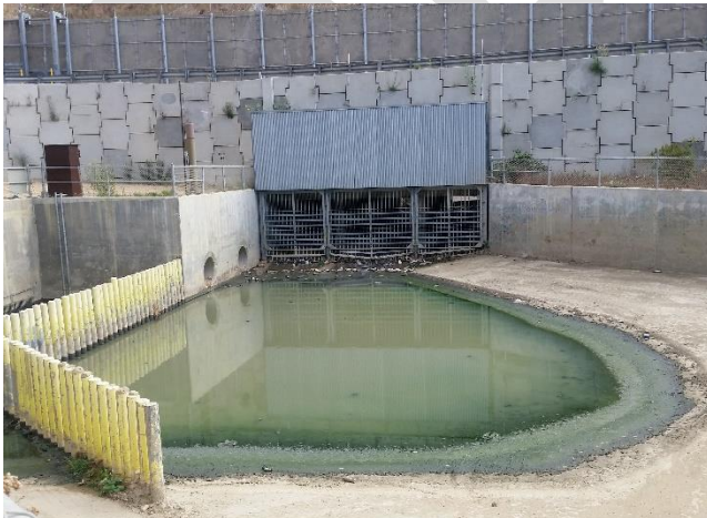
Wastewater pollution at Goat Canyon collector
