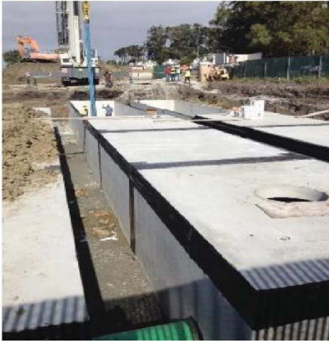
Figure 4. View of storage tanks during installation of the 2012 Wet Weather Flow Management Project
