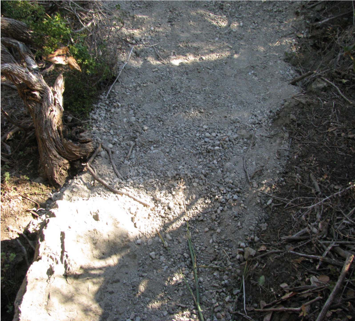
Photograph 3: Recent backfill of an erosion gully caused by the discharge.
