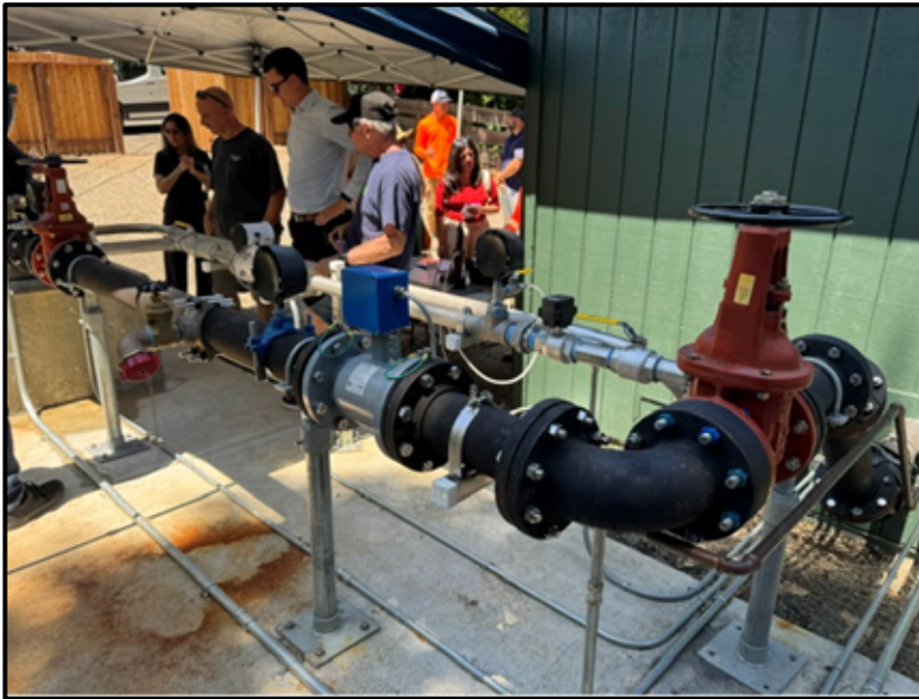
Photo 1: Park Avenue Aquifer Storage and Recovery facility can pump up to approximately 150 gallons per minute of groundwater.
