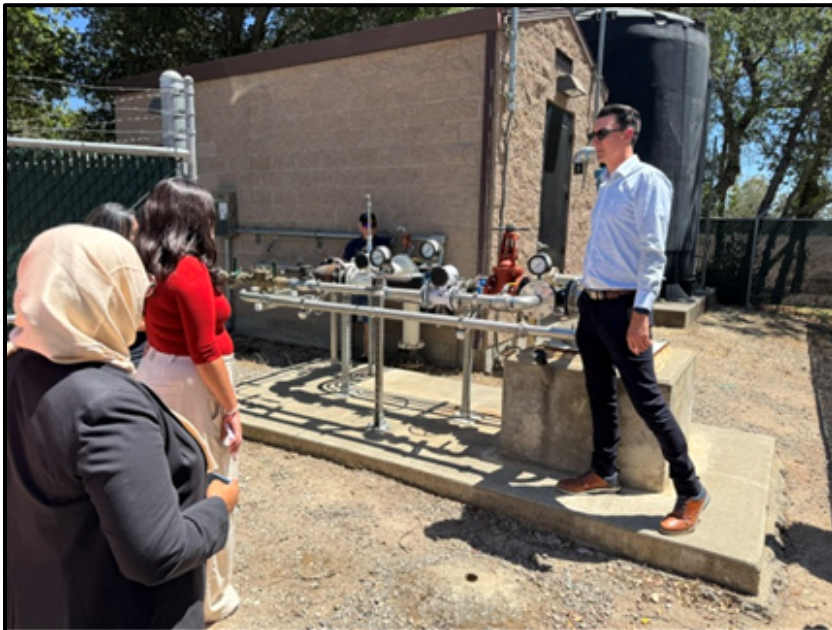
Photo 2: Verano Avenue Aquifer Storage and Recovery facility can pump up to approximately 200 gallons per minute of groundwater.
