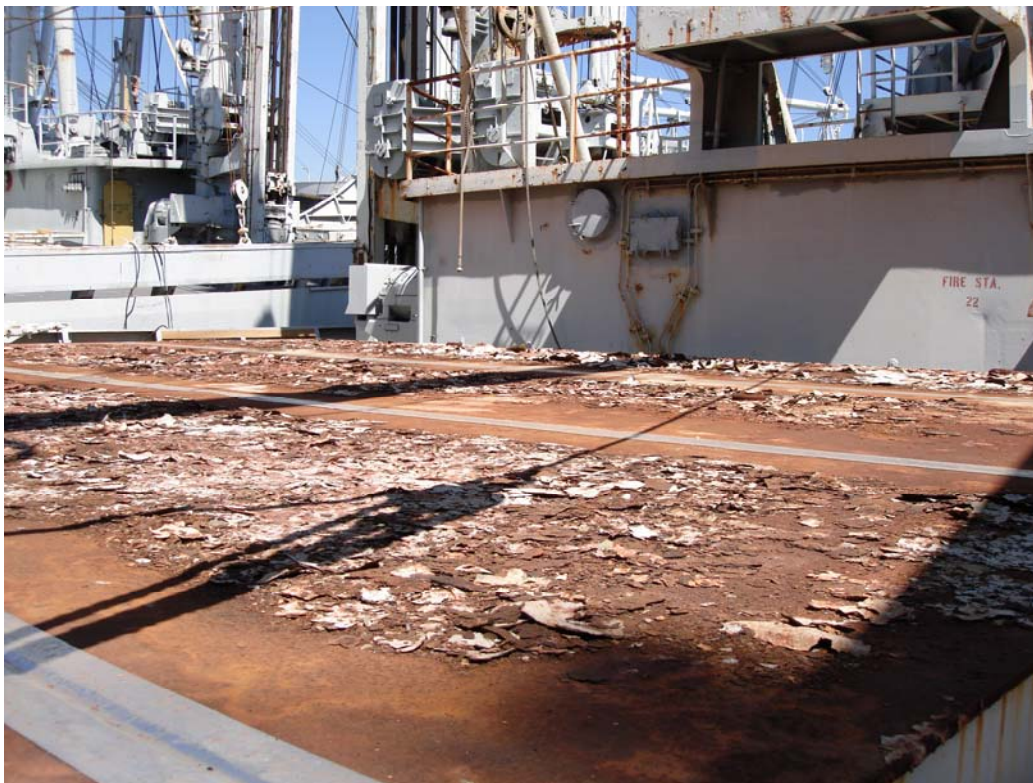
Photo #5 – Example of major paint exfoliation of a deck surface
