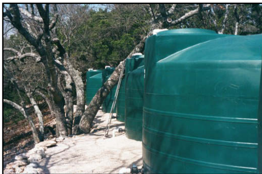
Figure 2-6. Low-profile 5,000-gallon polypropylene tanks
