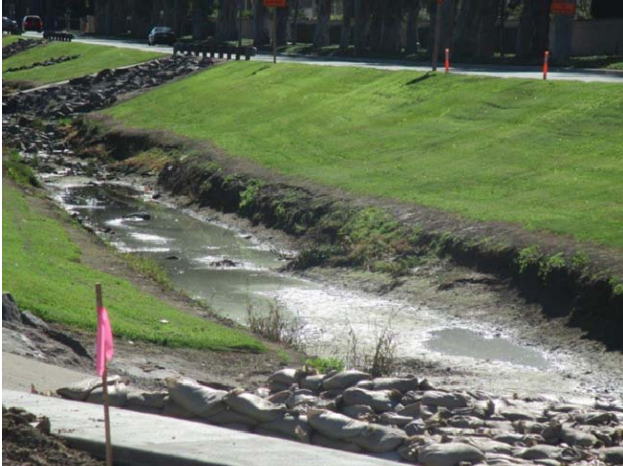
Figure 3. Central Irvine Channel near Culver Ave. looking upstream and showing mild channel erosion.
