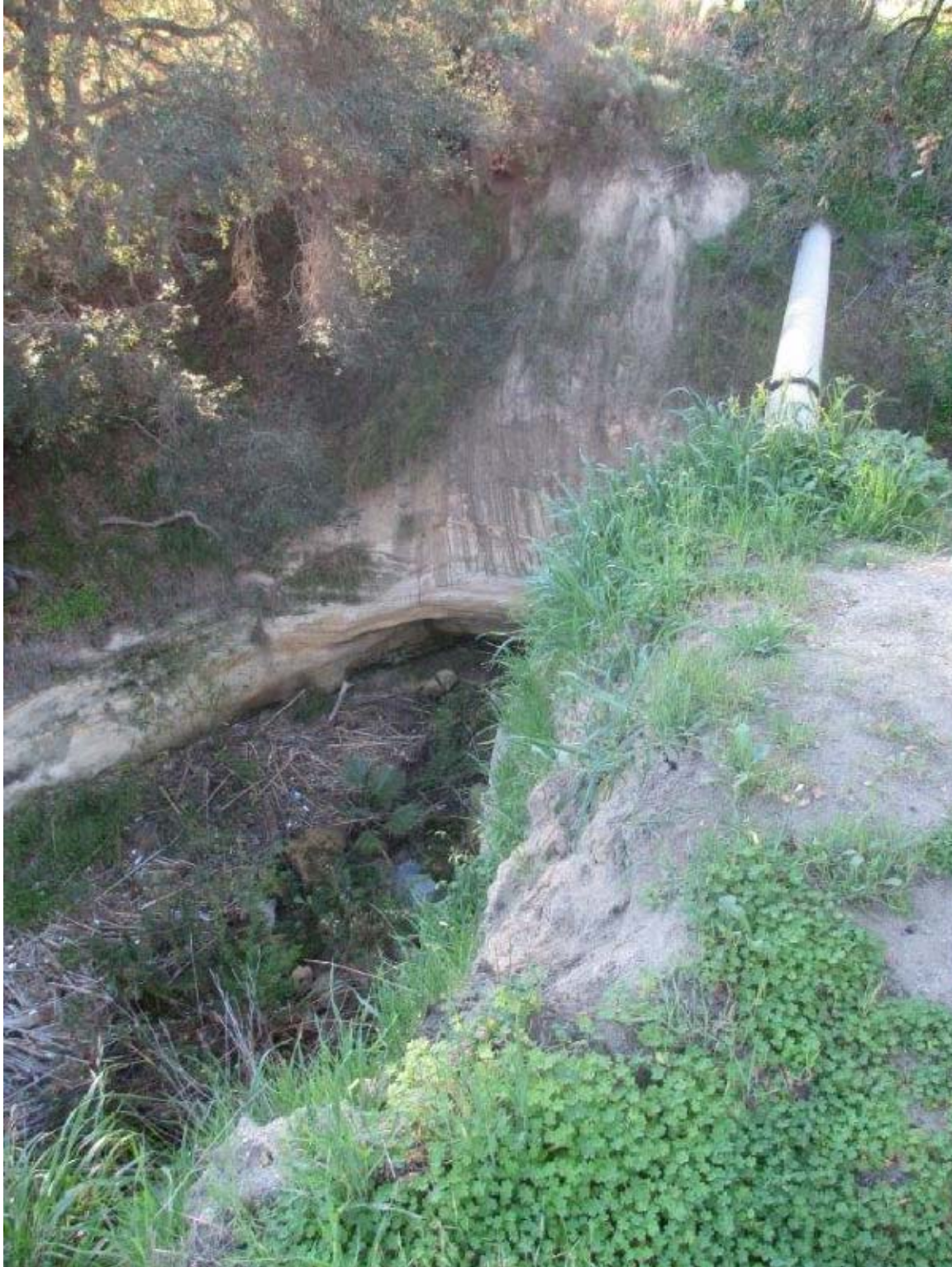
Figure 5. Serrano Creek a few hundred feet below Dimension Road looking over the top of a cliff into the canyon. The cliffs are 25-30 feet high and are undercut and unstable and are often just a few feet from the pedestrian trail which parallels the creek on the west side.
