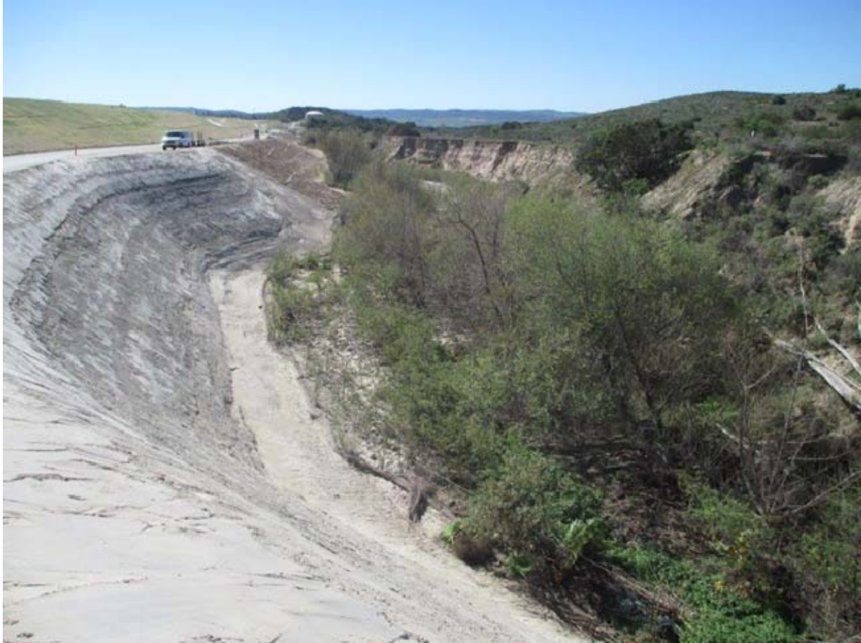
Figure 4. The Baker Ranch Gully looking downstream. The left bank on the Baker Ranch side has been smoothed and armored but the right bank on the U.S. government side has not been treated.
