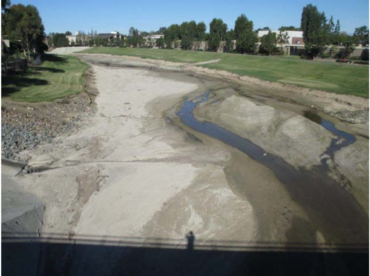
Figure 2. San Diego Creek between West Yale Loop and Jeffrey Road looking downstream and showing mild channel erosion. Note that the base of the grassed slopes is eroded away in some areas.
