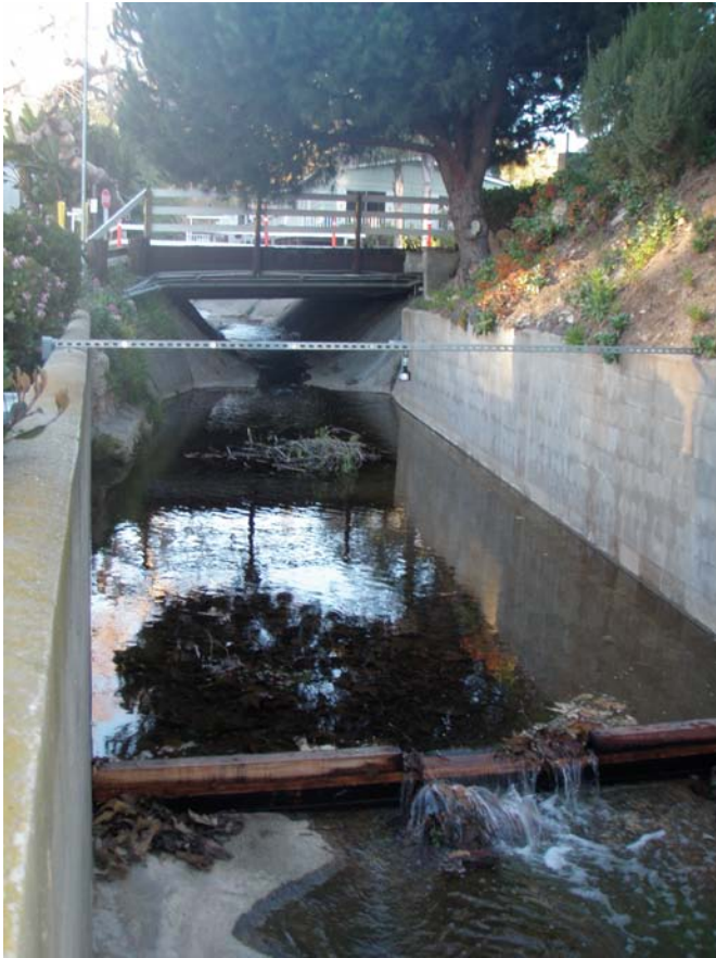
Figure 15. Ultrasonic Probe and Weir for Flow Monitoring
