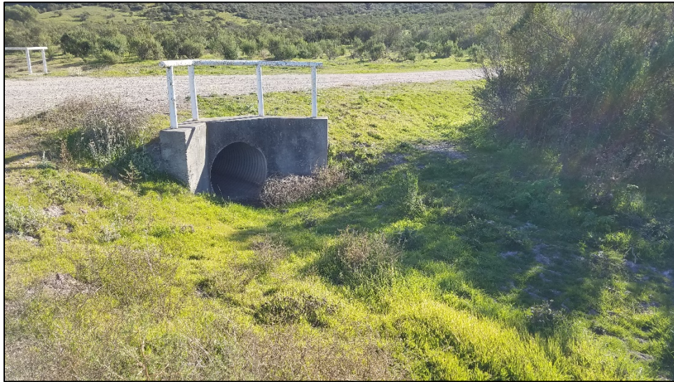
Photo A-1. View of Culvert 1 outlet from the Orcutt Hill Road shoulder. Photo taken February 10, 2020.
