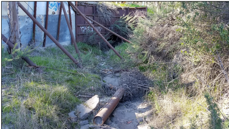
Photo A-6. View of the Culvert 5 inlet where Pine Canyon Creek flows under Orcutt Hill Road. Photo taken February 10, 2020.
