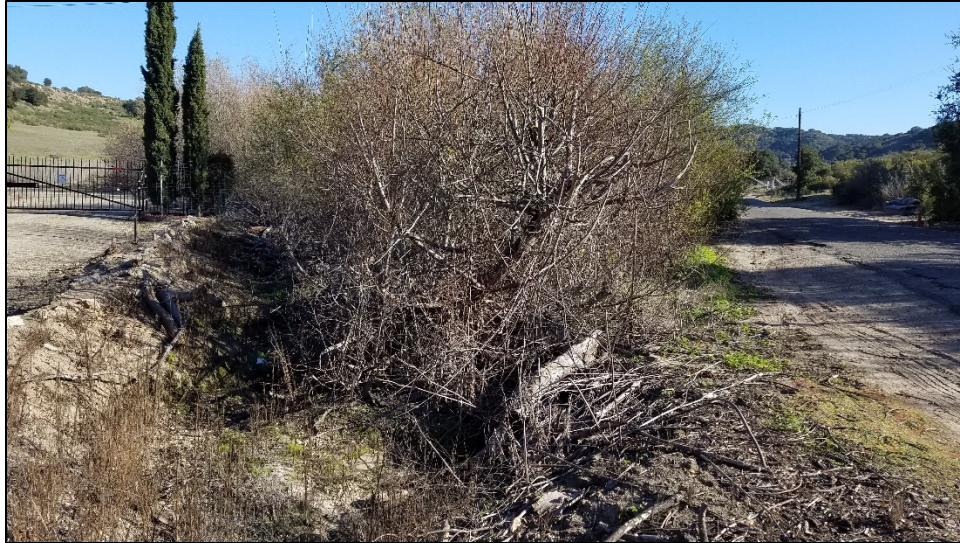
Photo A-3. View of the Unnamed Drainage at the Culvert 3 inlet. Photo taken May 19, 2020.
