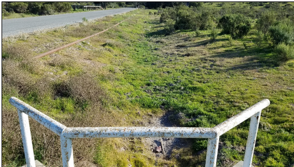
Photo A-2. View of the road shoulder at the Culvert 1 inlet. Photo taken February 10, 2020.
