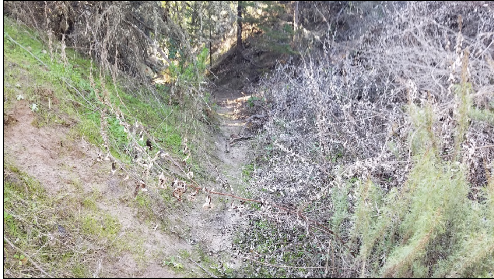
Photo A-5. View of the Unnamed Drainage channel immediately downstream of the Culvert 4 outlet. Photo taken February 10, 2020.
