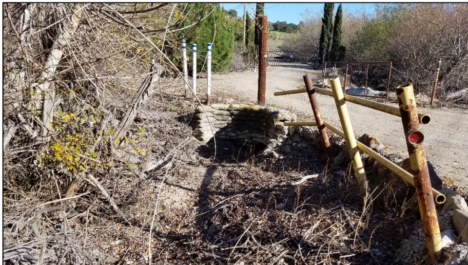
Photo A-4. View of the Unnamed Drainage at the Culvert 3 outlet. Photo taken May 19, 2020.
