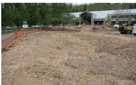
Green Infrastructure Stormwater Management
