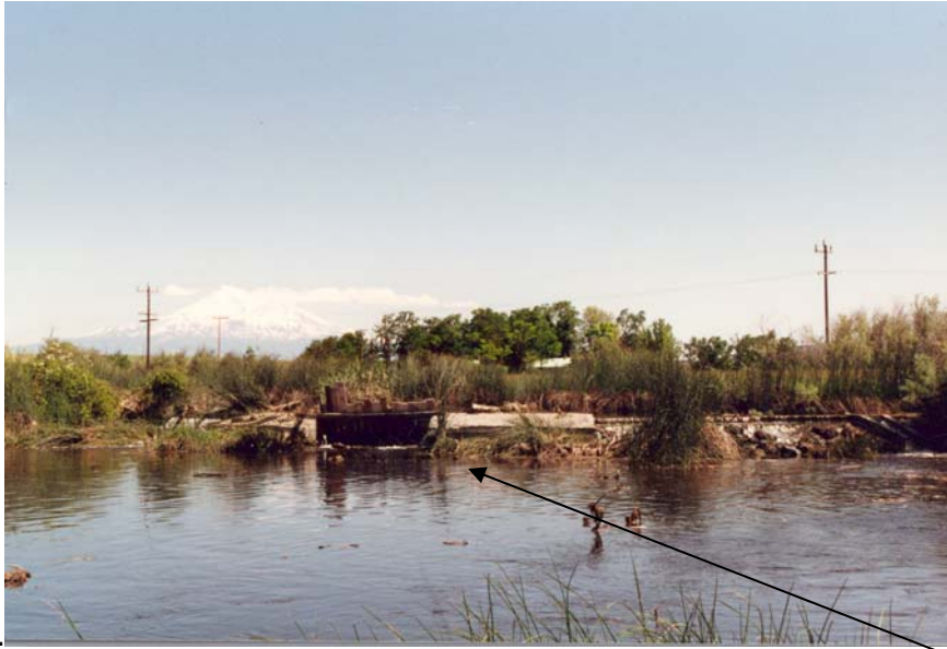
Small Dam, known as Araujo Dam, prior to removal from the Shasta River last October (2007)
